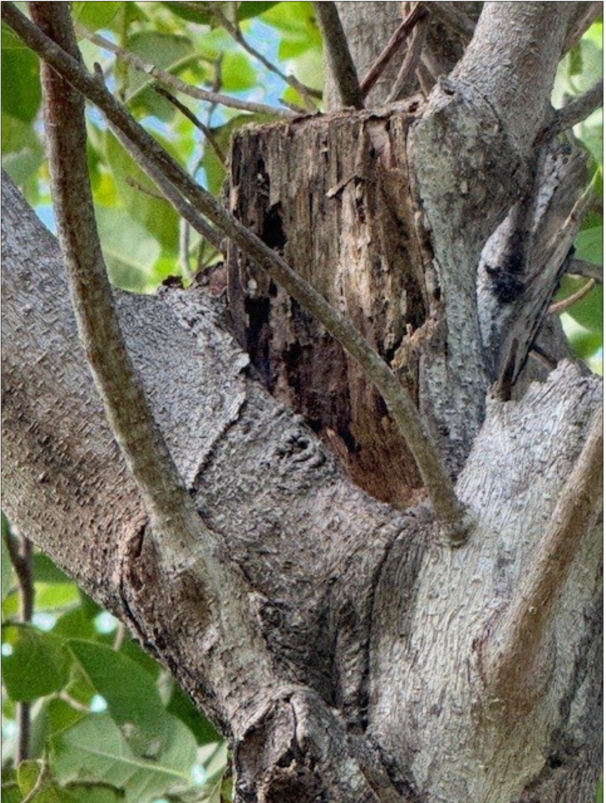
Aerial termite damage visible on high canopy limbs with improper pruning cuts visible.
