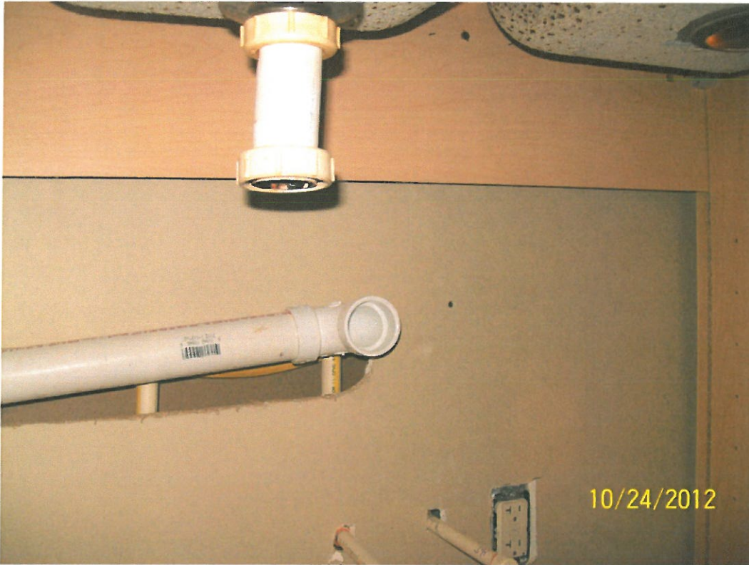
Open plumbing line. New electric socket installed. No permits for plumbing or electric on this date.
