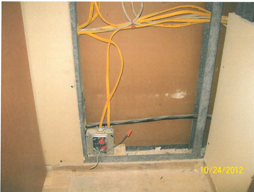
Further electrical installed to accommodate new kitchen appliances. No plumbing or electrical permits on this date.
