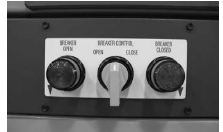
Devices Mounted on Secondary Terminal Compartment Door
