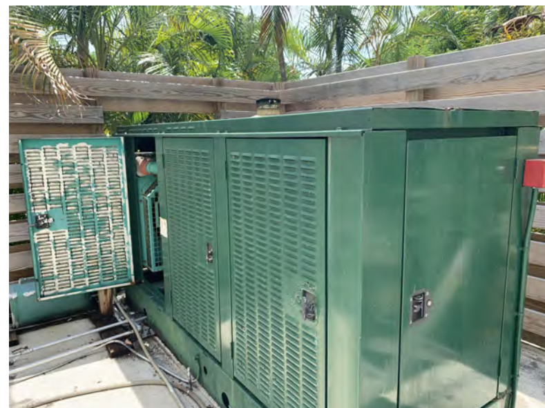
INSIDE THE EXISTING GENERATOR ENLOSURE
