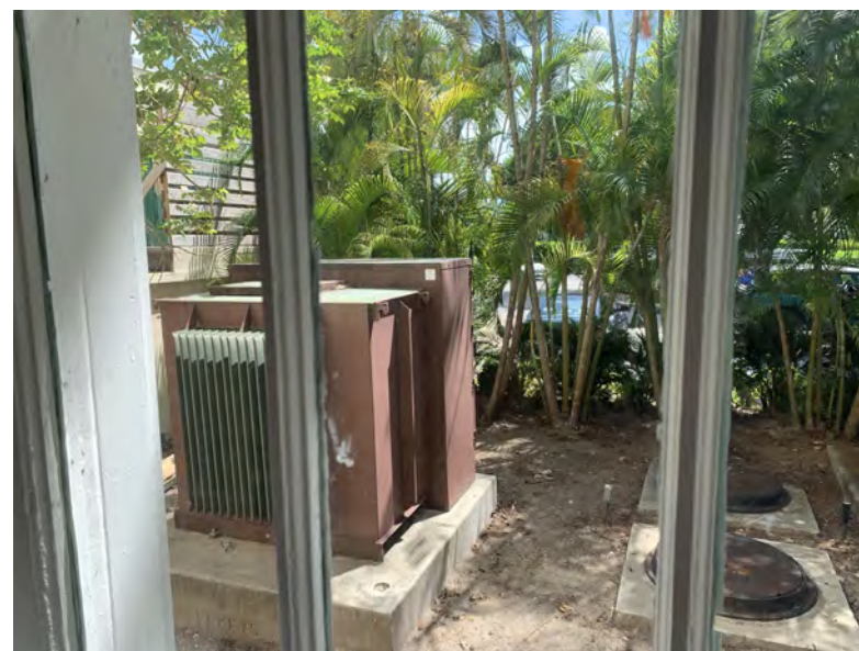
VIEW OF TRANSFORMER AND CISTERN FROM INSIDE BUILDING
