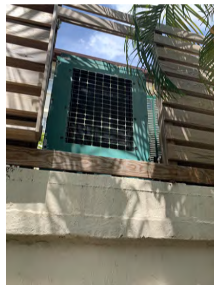
EXISTING GENERATOR VENT
