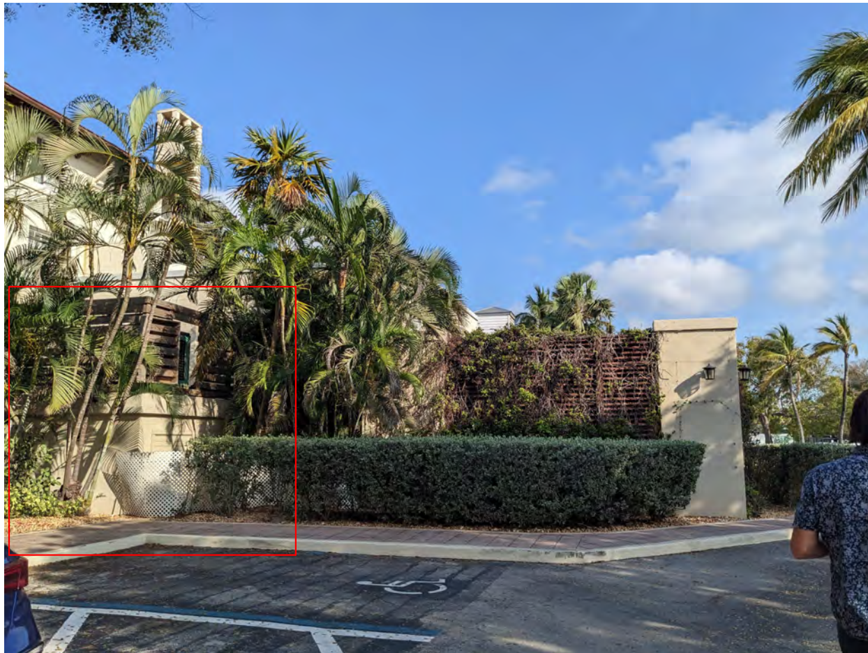
VIEW OF GENERATOR AND PLATFORM FROM PARKING
