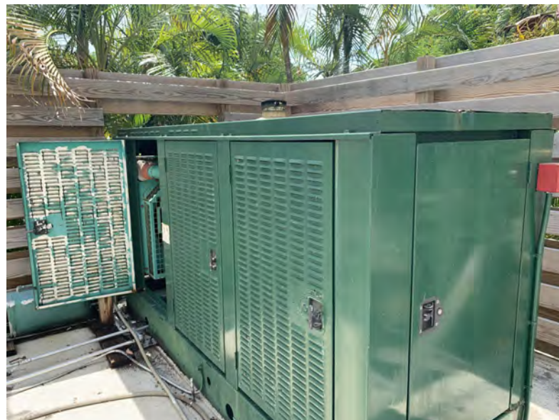
INSIDE THE EXISTING GENERATOR ENLOSURE
