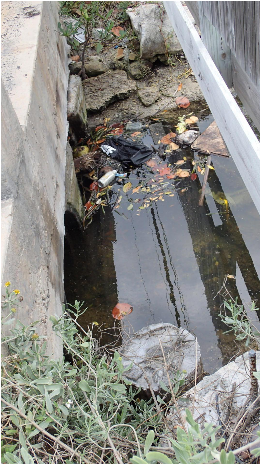
Photo of culvert at Northside Drive showing debris accumulation and blockage into the pipe
