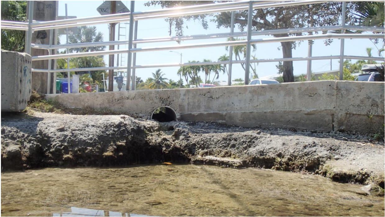
Photo of a stormwater outfall into the Riviera Canal showing a partial obstruction in the pipe.
