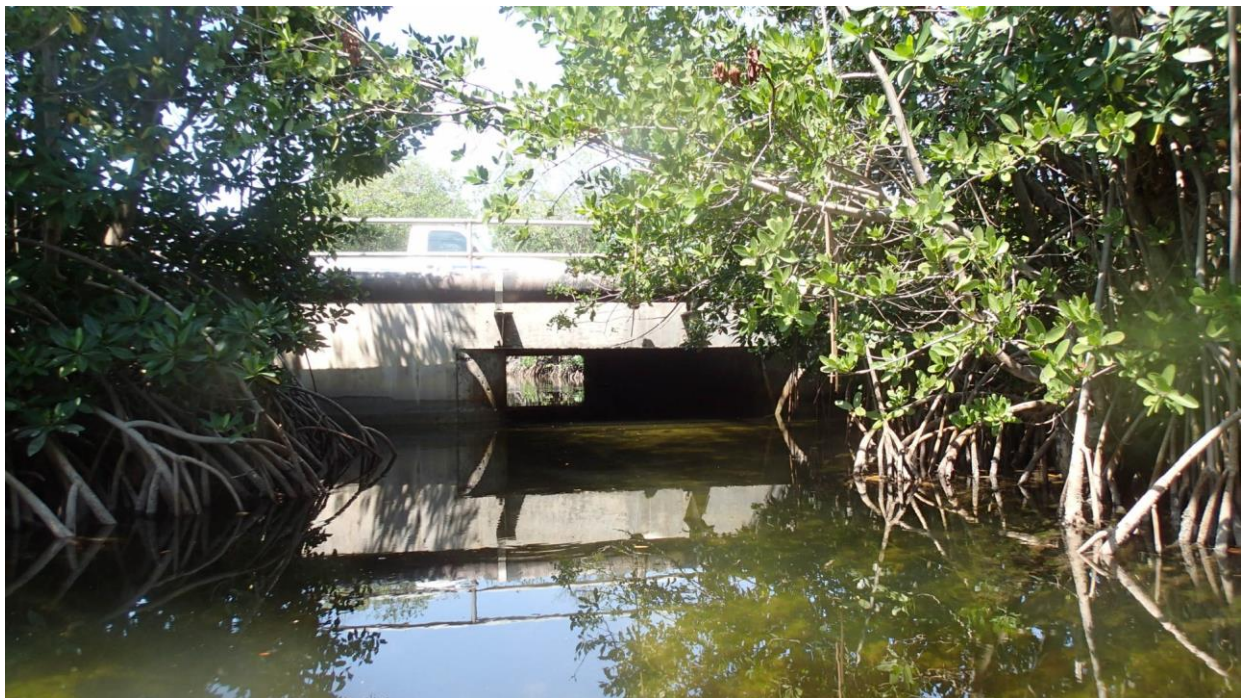
Photo of the Riviera Canal at Flagler Avenue showing mangrove branches and roots encroaching into the conveyance.
