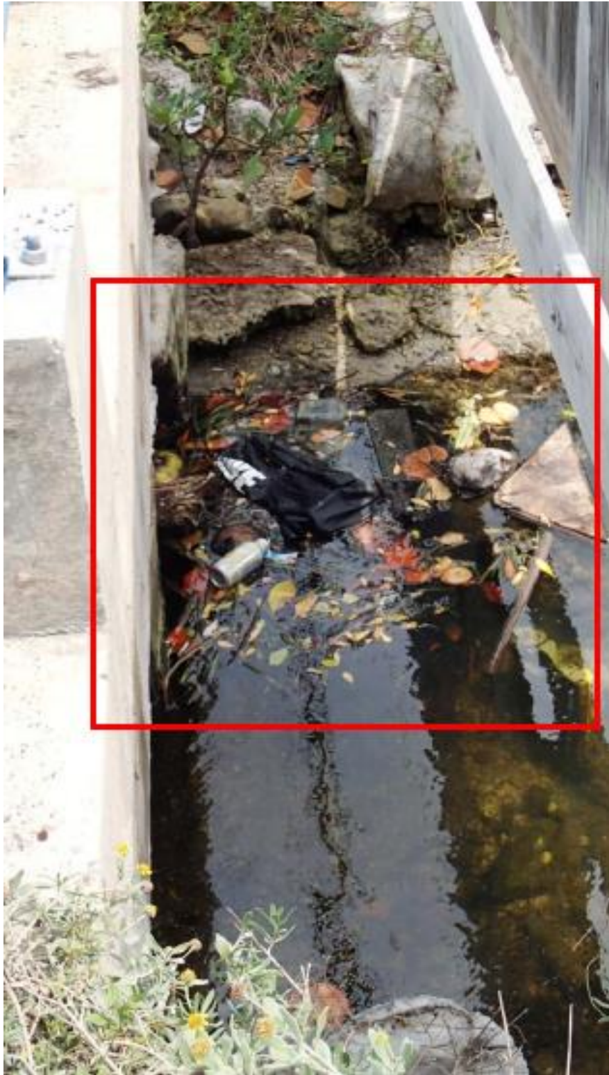
Photo 1. Debris blocking flow through culvert. Debris should be removed and disposed of properly per City of Key West regulations.
