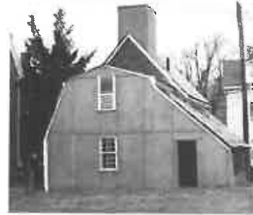
Temporary stabilization or "mothballing" with materials, such as plywood and building paper, can protect the roof of a project until it can be properly repaired or replaced. Photo: NPS files.
