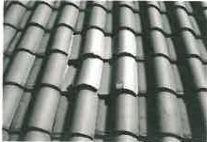
Repairs on this pantile roof were made with new tiles held in place with metal hangers. Photo: NPS files.
