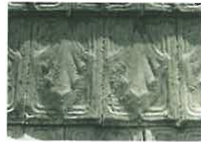
Tin shingles, commonly embossed to imitate wood or tile, or with a decorative design, were popular as an inexpensive, textured roofing material. Photo: NPS files.
