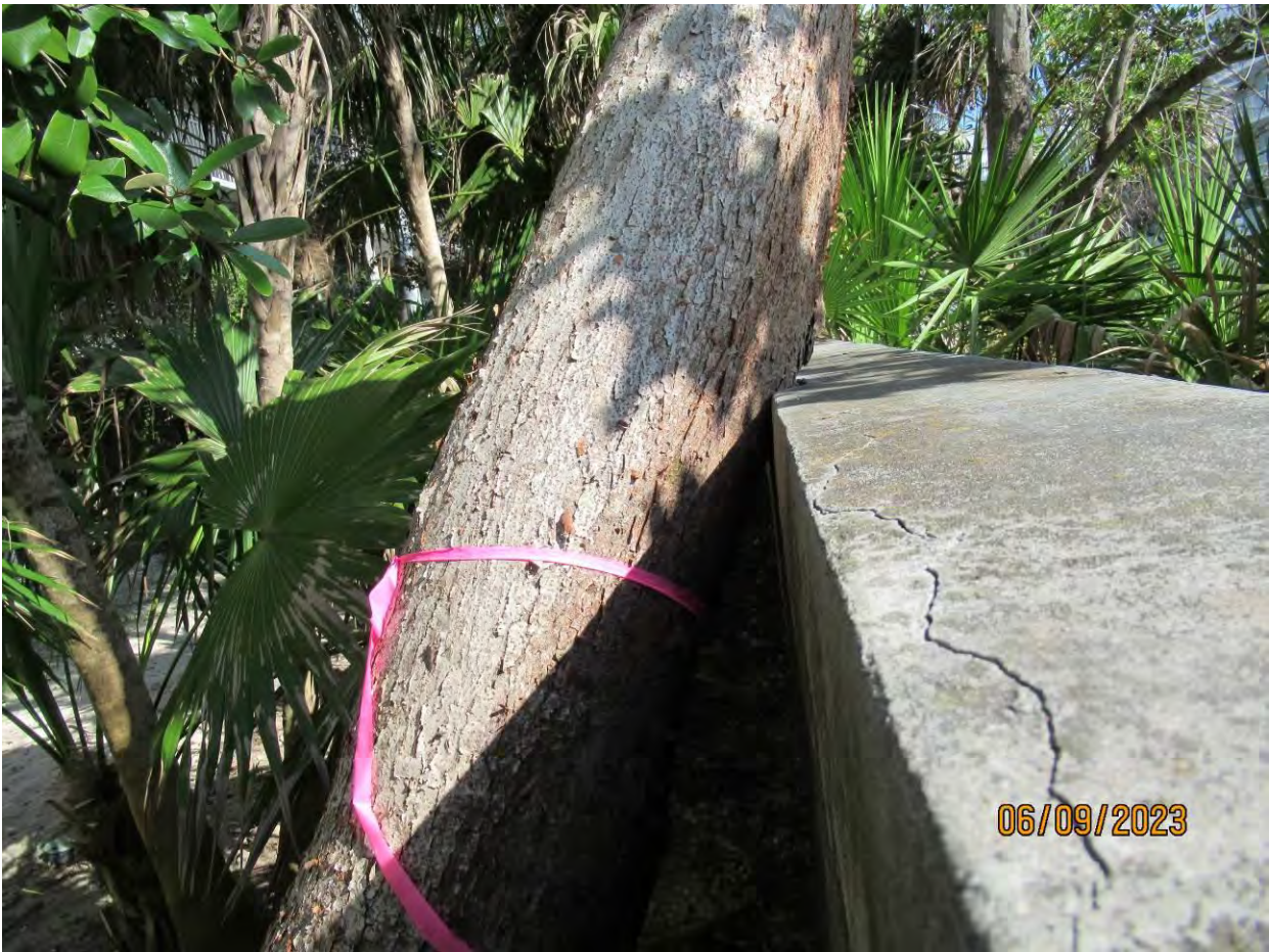
Two photos showing tree trunk against concrete wall, view 1.
