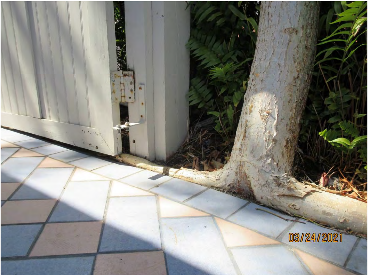
Photo of base of tree and root structure. Note main structural root growing under gate.
