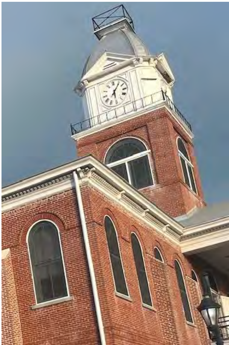
Detail of windows coverings and tower deterioration and missing parts.
