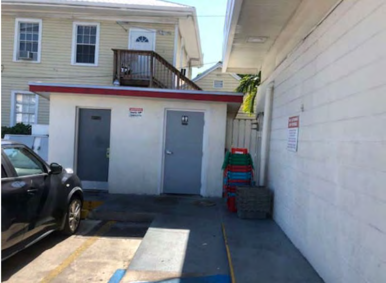
Exterior bathrooms to be relocated inside and made to be ADA compliant.
