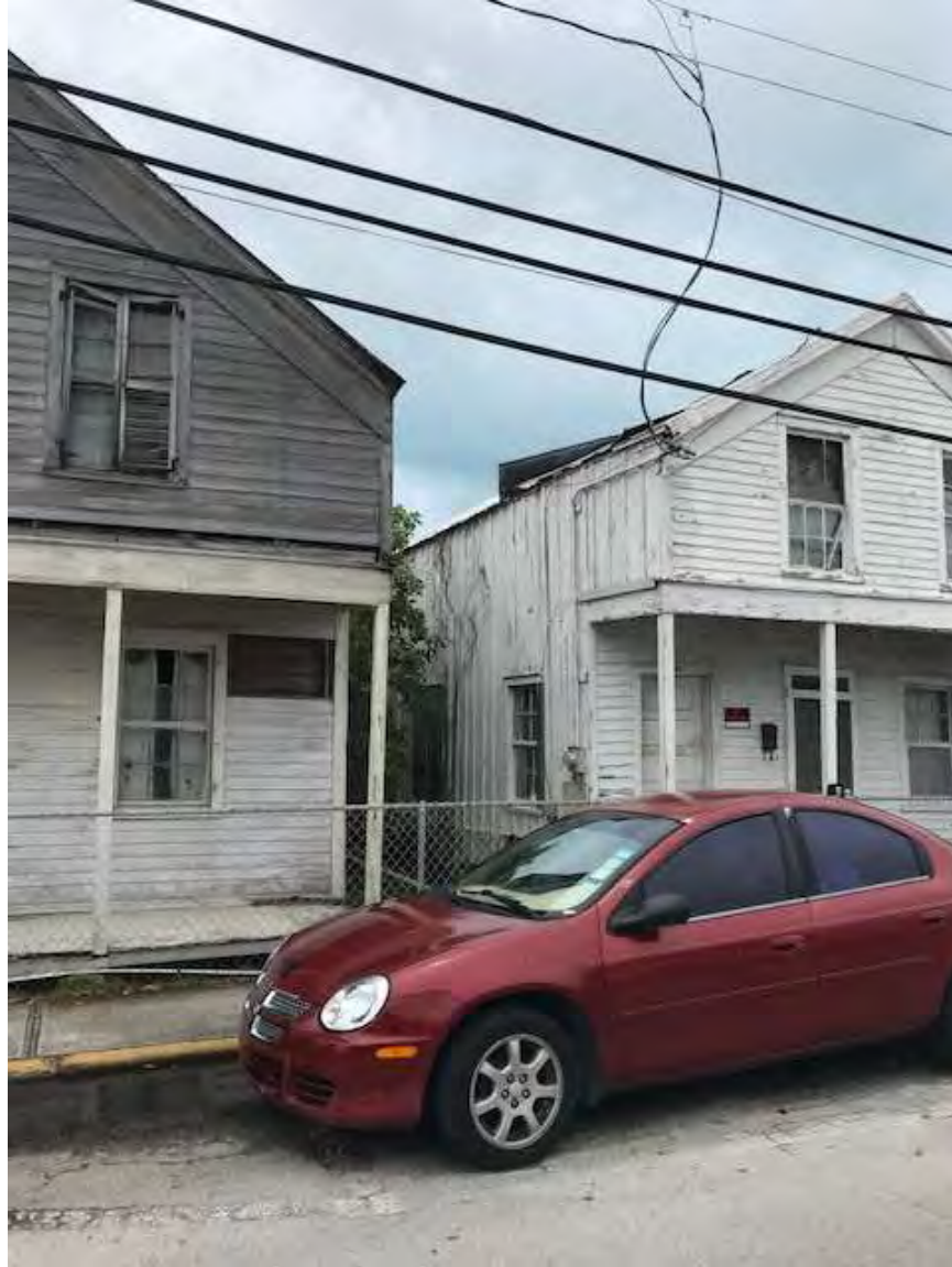
1010 Olivia Street right side of the photograph. Proposed skylight will be visible from Olivia Street.
