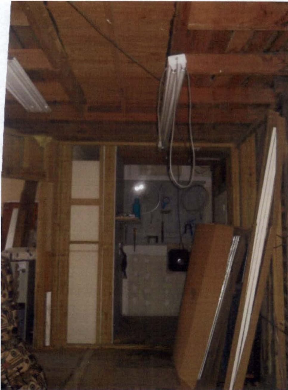
The end of this hall is where we had to open the wall to the rest (back) of the house...
