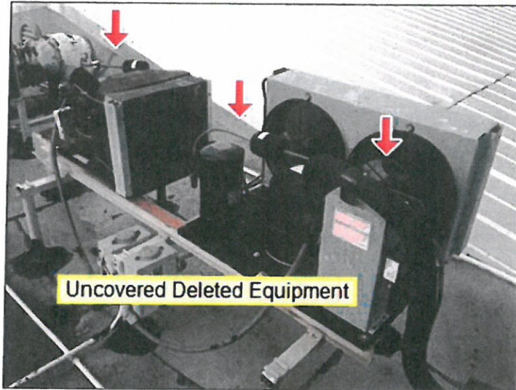
9.0 Picture 4 Equipment On Roof
