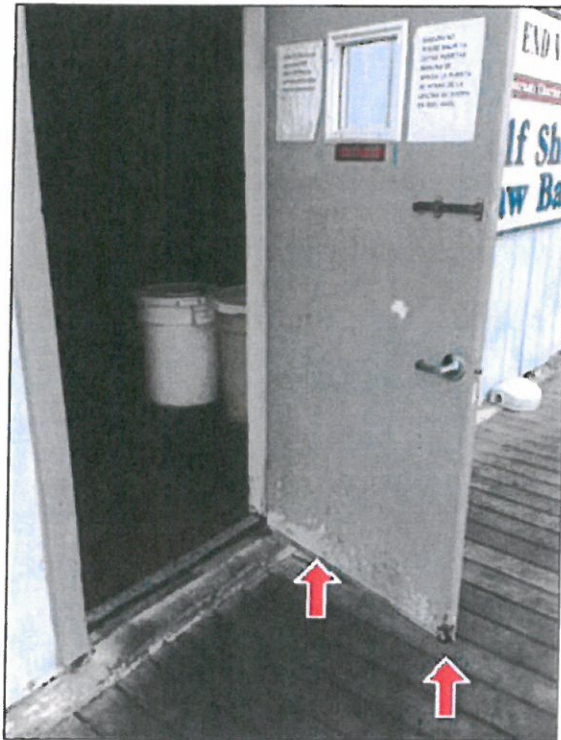
2.1 Picture 5 Typical Damaged Exterior Door
