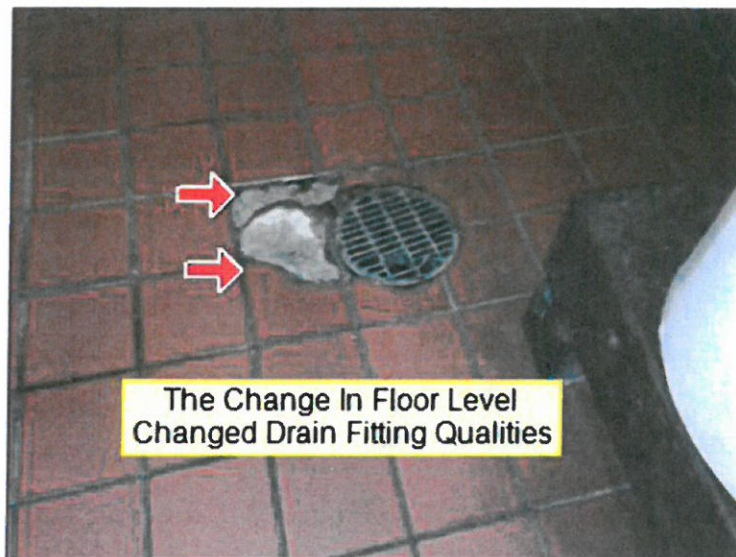
4.0 Picture 2 Kitchen Drain System
