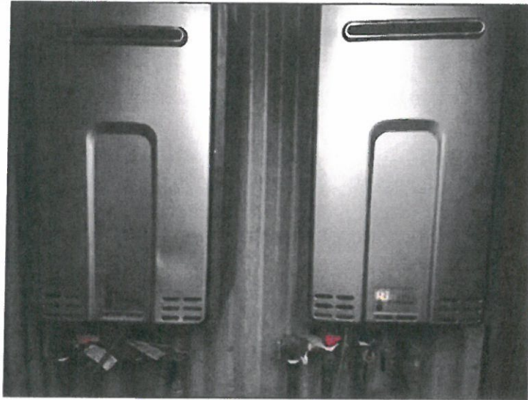
4.2 Picture 1 2 Tankless Units
