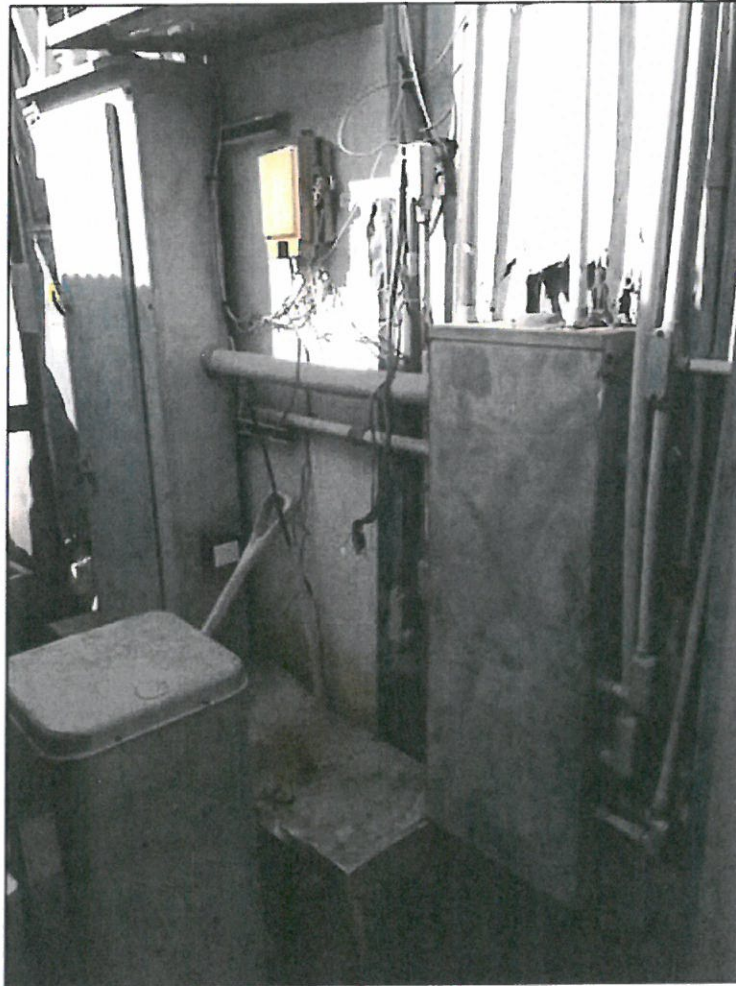
8.1 Picture 1 Underground Service Entrance
