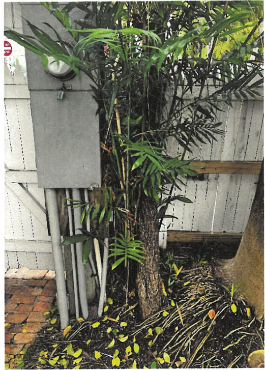
#9 Buttonwood – conflict with electrical
