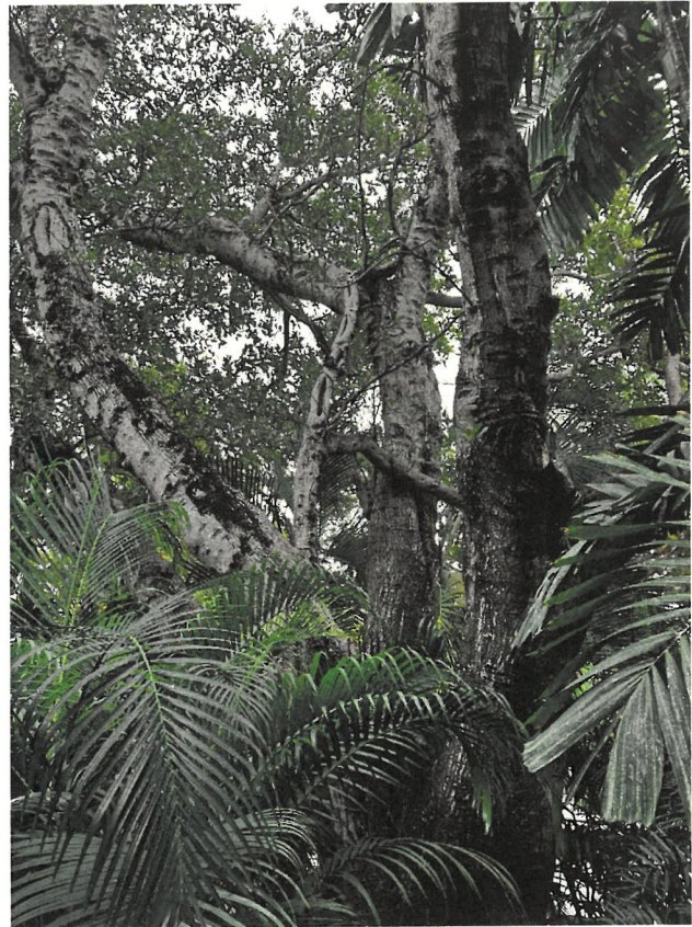
# 1 Strangler Fig – Conflict and under mining House
