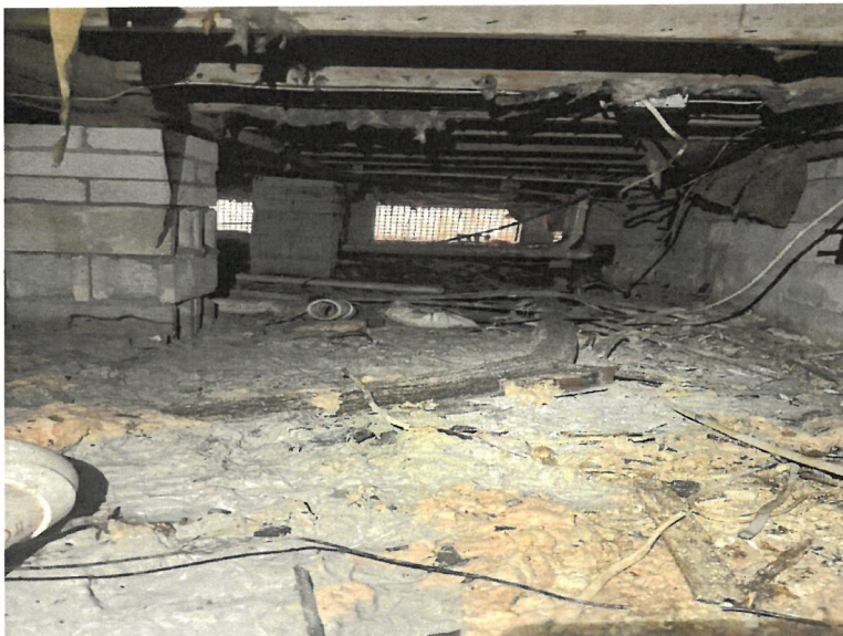
# 1 Strangler Fig – Conflict and under mining House foundation
