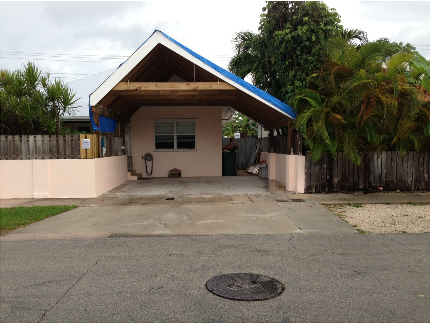
Newly Constructed Carport with large roof surface area and zero set-back from adjoining property.
