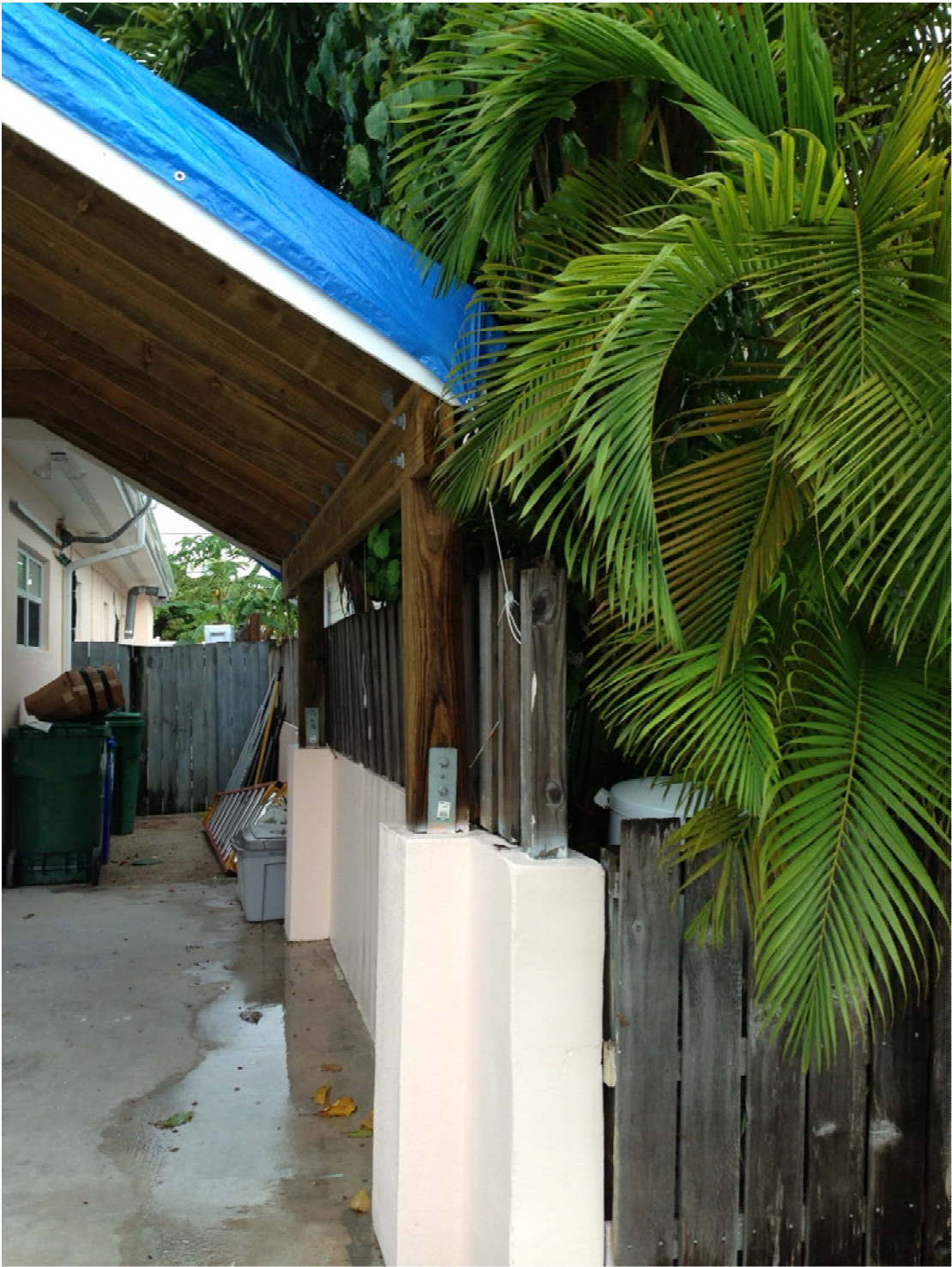
Proposed gutter hangs over fenceline.
