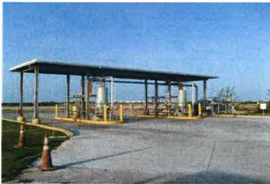
Jet Fuel Pump Station, Boca Chica NAS
