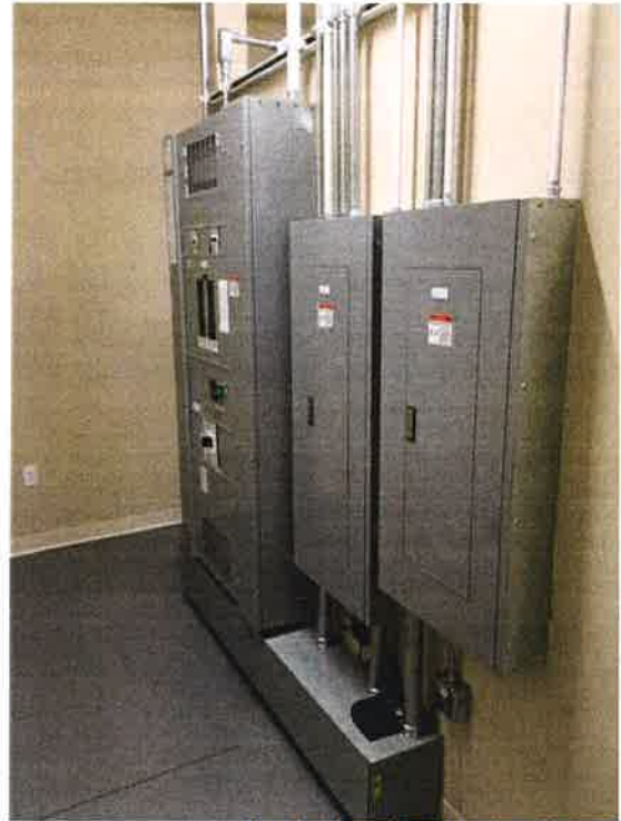
Electrical Panels at Marathon City Hall
