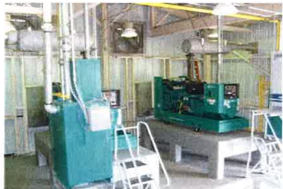
USAF, Generators & Switchgear, Cudjoe Key, FL
