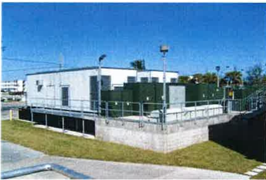
JIATF South, Emergency Generators (1.5 MW)
