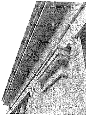
Close up of exterior of Building A, showing the columns and cornice line at the top of the wall. Elements such as this are rare in today's buildings, as they are expensive to build.
