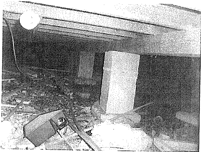
Typical interior foundations at Building A. The wood framing, seen at top, bears on girders, which in turn bear on concrete pier footings. All debris under the building should be removed, and damaged girders and framing should be sistered with new material, or replaced.
