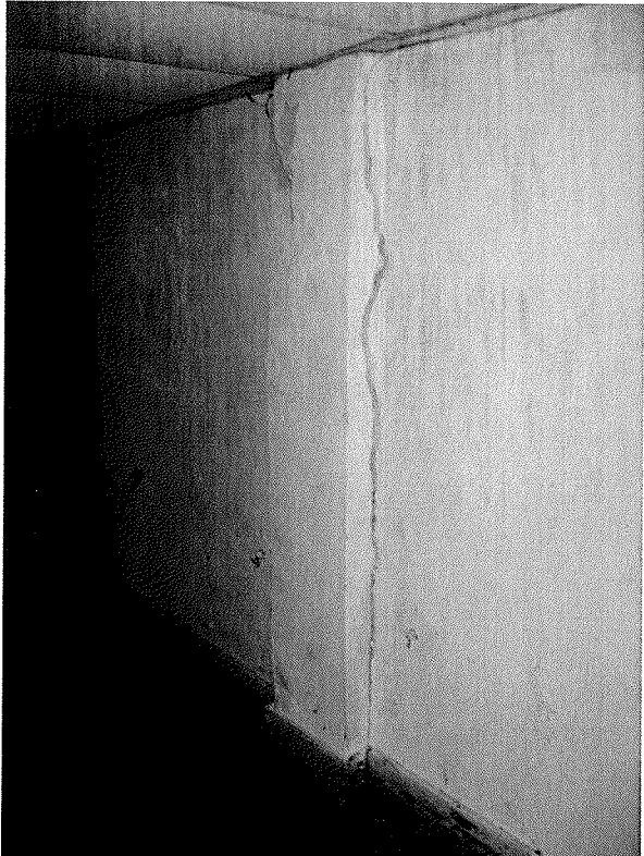
Photo of existing spalled concrete column at inside of building, along exterior wall. Note crack at wall-column joint. Contractor to repair spalling at all tie beams and columns and patch stucco. These columns are located under each wood truss, and are marked RC2 on Structural Plan S1.1. See repair detail, sheet S2.1. See structural details and specifications.
