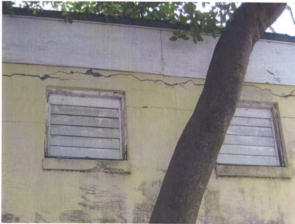
Detail photo of 2 nd floor spalling tie beam at north façade. Contractor to repair spalling at tie beams and columns and patch stucco. See structural details and specifications.
