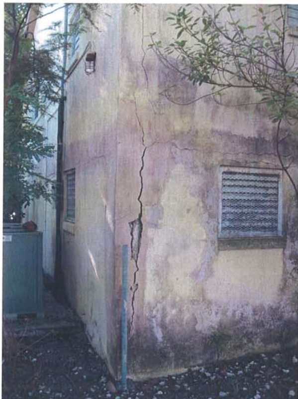
Detail photo of spalling at NE corner of building. Contractor to repair spalling at tie beams and columns and patch stucco. See structural details and specifications.
