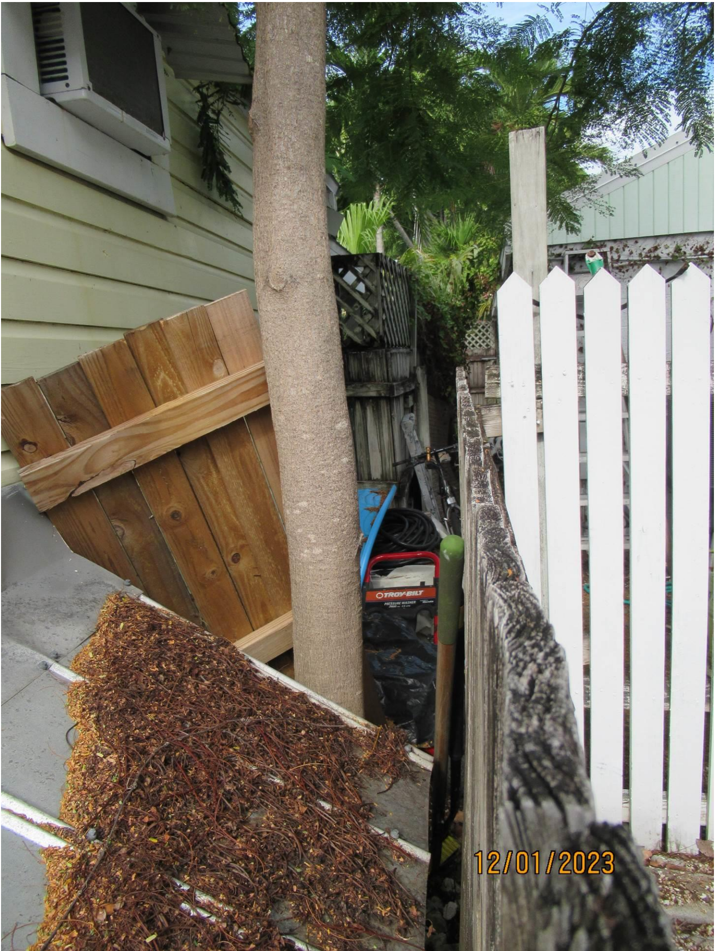
Photo of tree trunk showing location between fence and structure.
