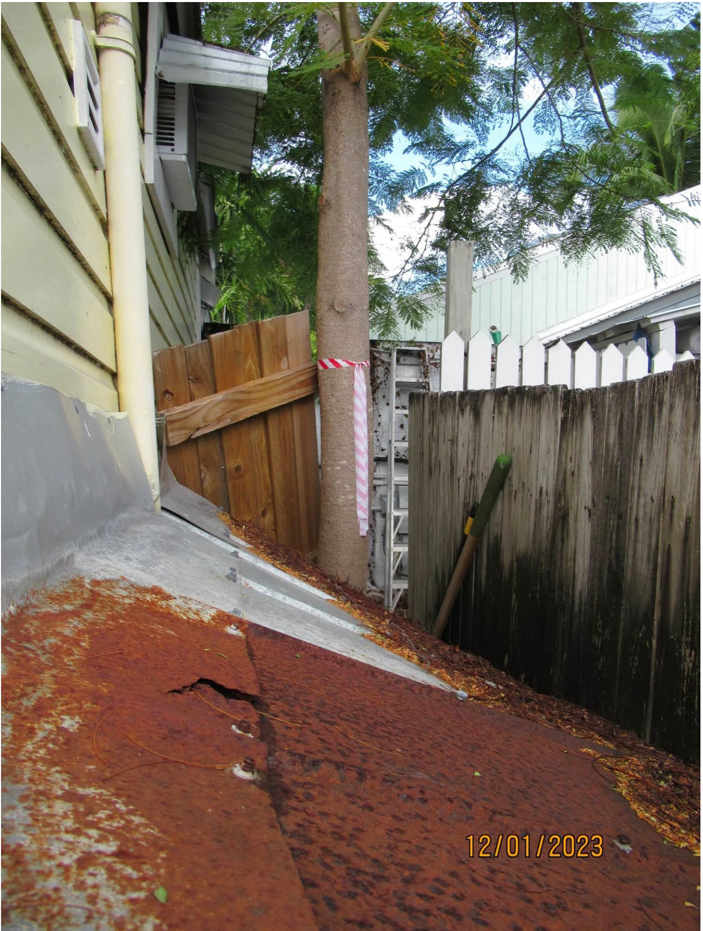
Photo of tree trunk and canopy in relation to structure, view 3.
