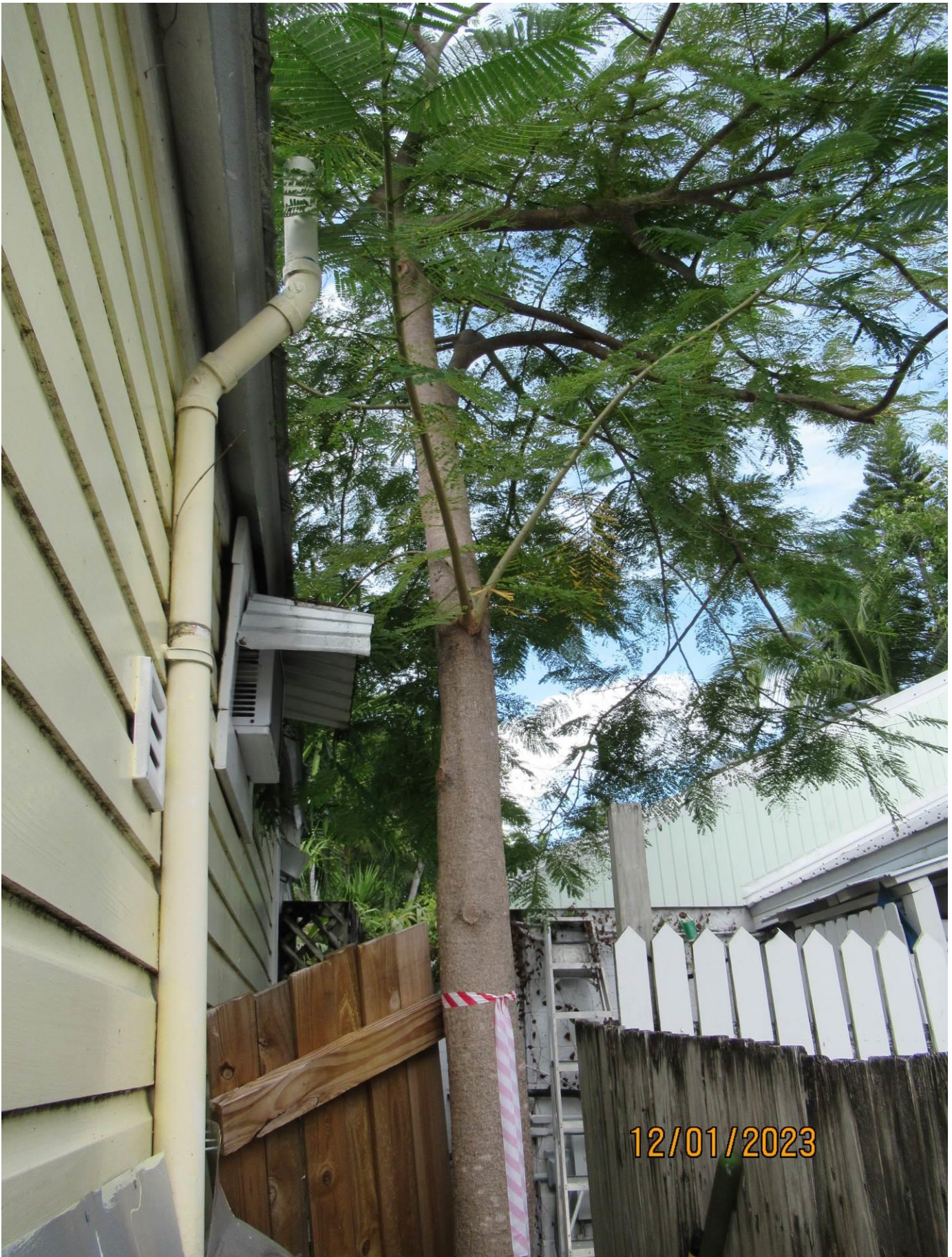
Photo of tree trunk and canopy in relation to structure, view 2.
