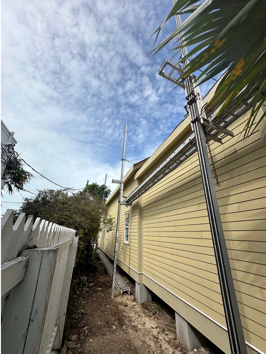
South side of house that faces Fausto's looking from the back of the lot. The Shed Dormer will be on this side. There will be landscaping so that you cannot see the house or shed dormer from Fausto's.
