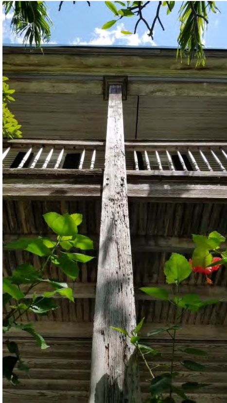
Existing front porch column. Note severe deterioration and missing guardrail spindles. Patch and paint column and siding. Repair existing column. Paint.
