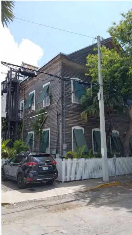
General View of NE corner of building. Repair all deteriorated siding. Paint building white and install sealant. Repair deteriorated columns, guardrails and porch decking. Refinish all wood shutters in stained wood.
