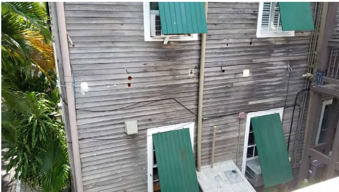
Damaged and deteriorated siding at north side of building (rear). Patch and paint siding. Remove all abandoned conduit. Patch and paint existing windows. Refinish all wood shutters in stained wood.
