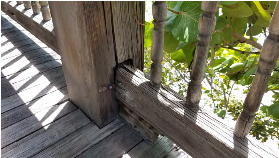
Detail of damaged column at 2 nd floor porch. Column wood is checked. Guardrail is loose. Repair in kind. Paint porch decking. Paint columns and guardrail. Repair wood in kind.
