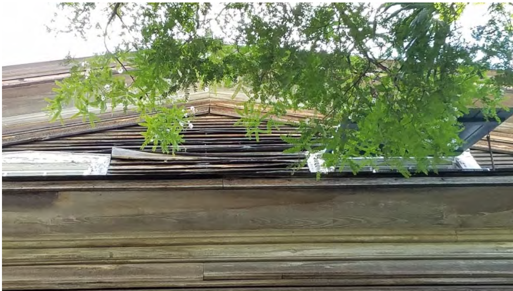
Detail view of severely deteriorated siding at west gable. The siding is so deteriorated that water and air intrusion is occurring.
