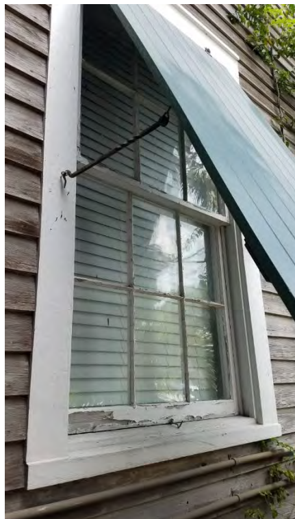
Detail view of existing historic putty glazed window. Patch and paint existing putty glazed DH window. Refinish all wood shutters in stained wood. Shutter types vary. (Wood Louvered and Wood Bahama style. )
