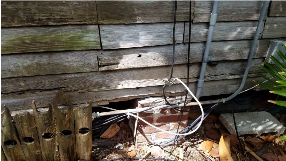
Deteriorated siding at east side of building. Patch and paint existing siding. Remove all abandoned conduit.
