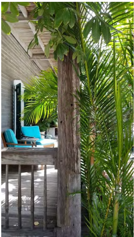
Existing porch column at SW corner of porch. Column is extremely deteriorated. Repair all deteriorated siding. Paint building white and install sealant. Repair deteriorated columns, guardrails and porch decking in kind.
