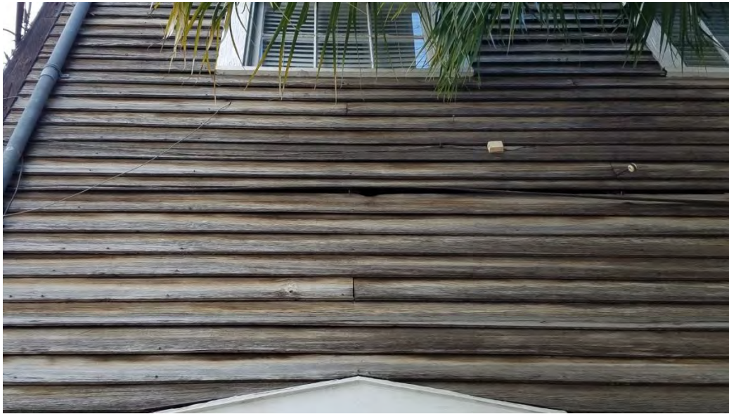
Detail view of existing damaged siding at west façade.
