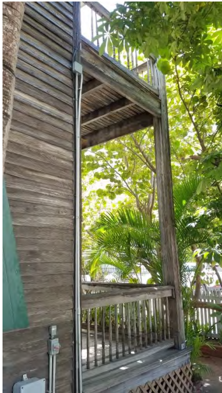
Side view of existing front porch. Repair all deteriorated siding. Paint building white and install sealant. Repair deteriorated columns, guardrails and porch decking in kind. Remove all abandoned conduit.
