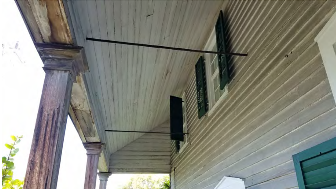
View of ceiling at 2 nd floor porch. Note traces of white paint.
