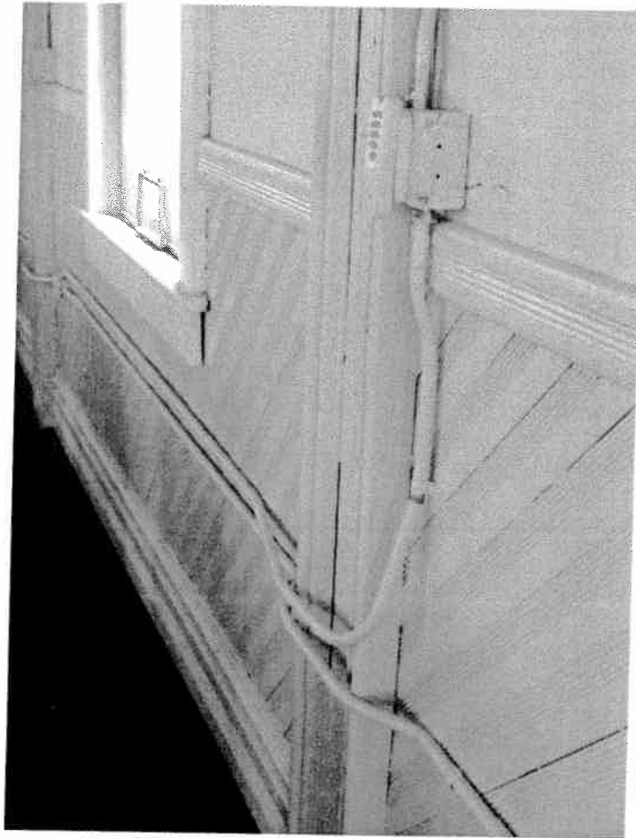
Figure 51 Conduit on Woodwork
