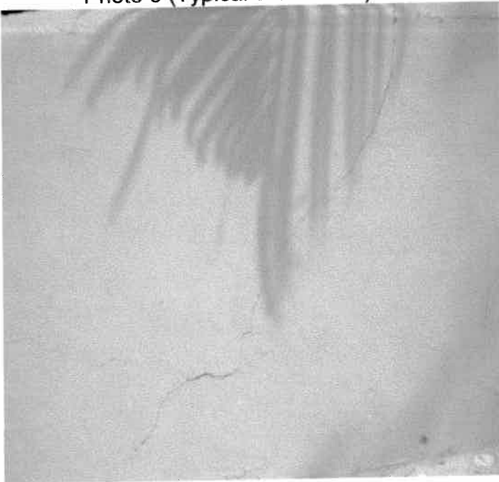
Photo 3 (Typical Wall Crack)
