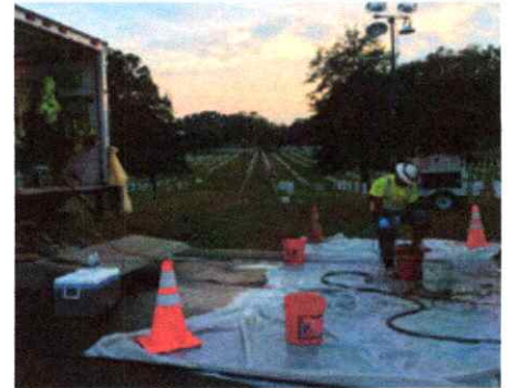
Determining the exact location of sewer assets and evaluating their condition is a complete process in planning for rehabilitation.
