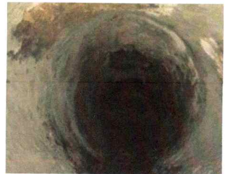
Existing RCP pipe with initial patches to stop active infiltration.
