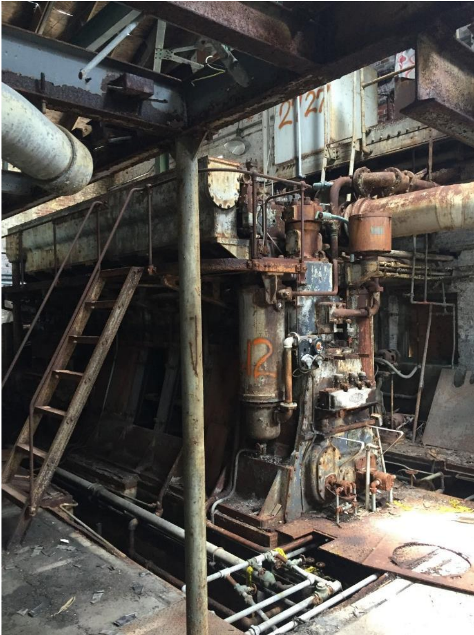
PHOTO 2: Inactive generator inside buildings at the Site
