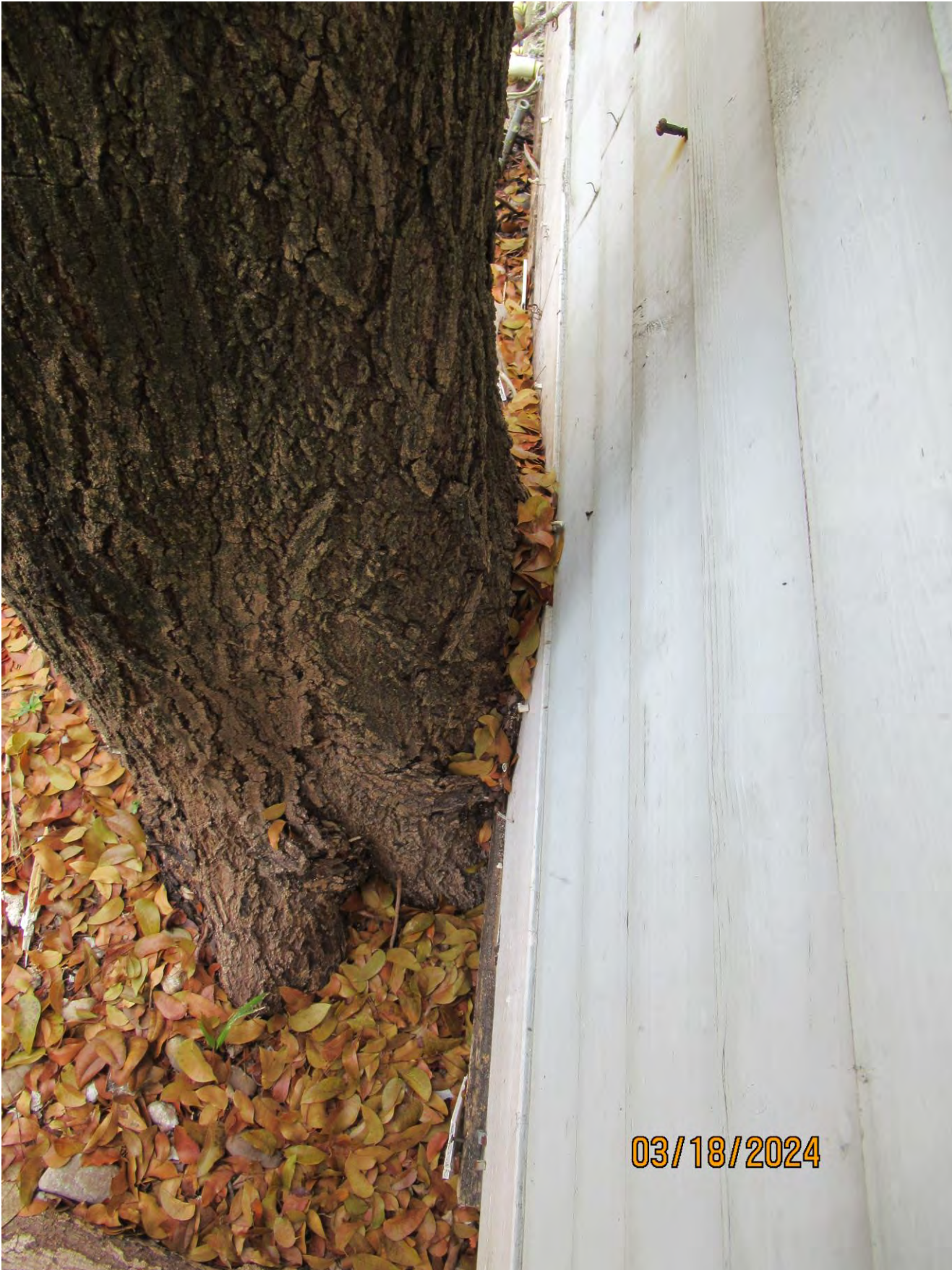
Photo showing base of tree against house.
