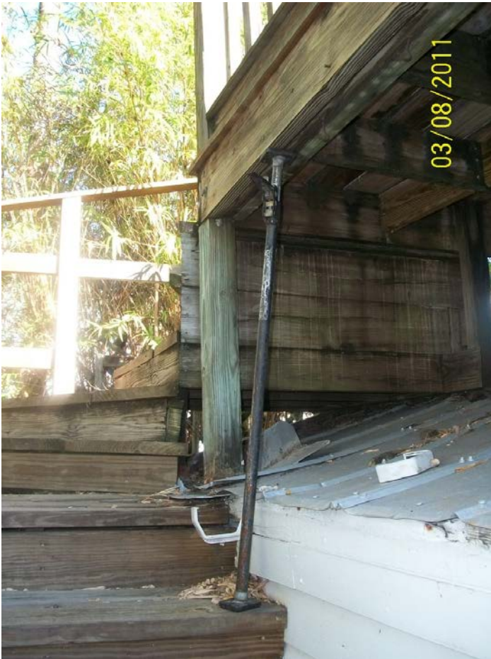
back balcony jacked up
