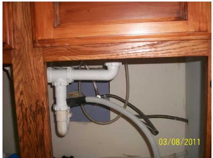
plumbing for newly installed dishwasher
