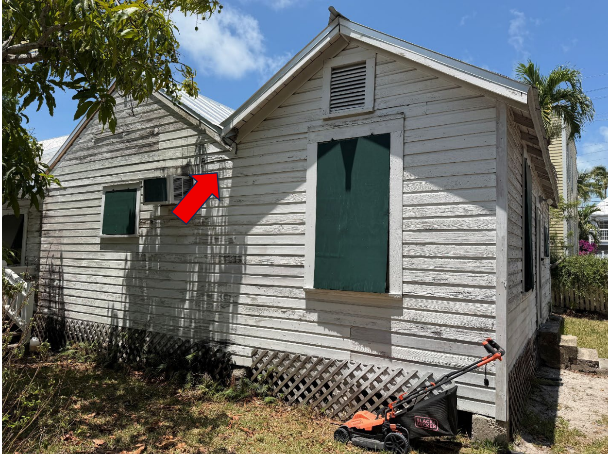
Figure 4 - South Side - Sawtooth additions. Engineering area of concern is FFL to beam clearance if roofline is not modified
