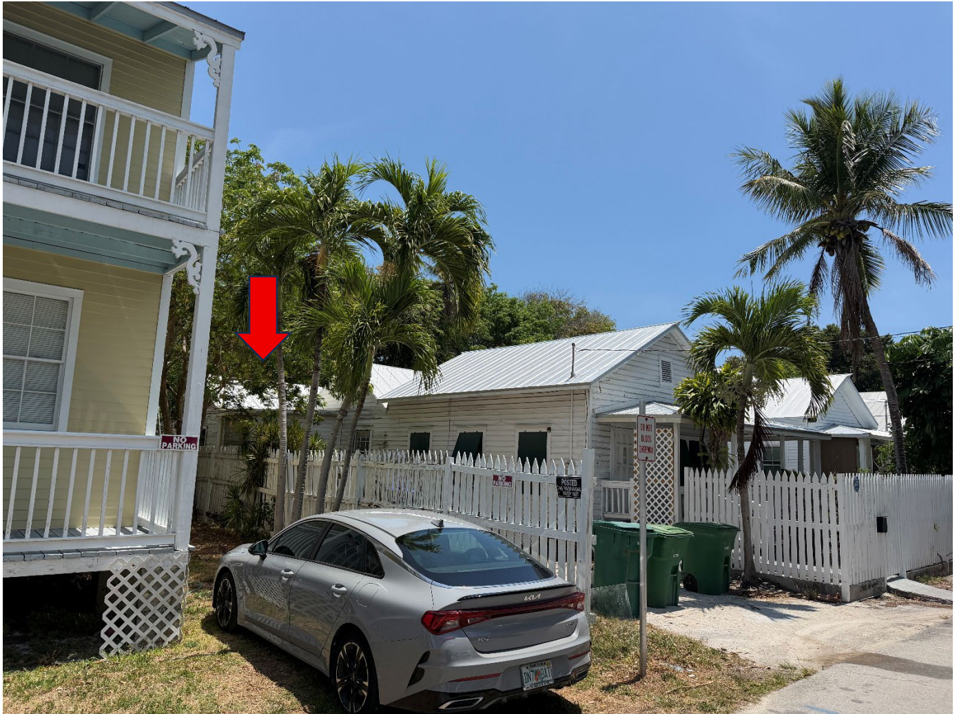
Figure 2 - Street View – North Side. Existing flat roof is shown with red arrow.
