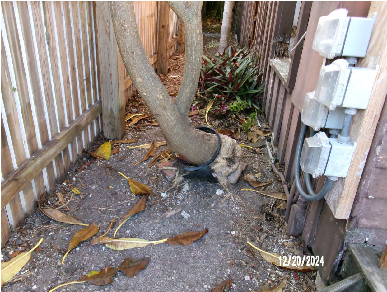
Photo of base of tree, view 1. Tree appears to have grown from pot and into the ground.
