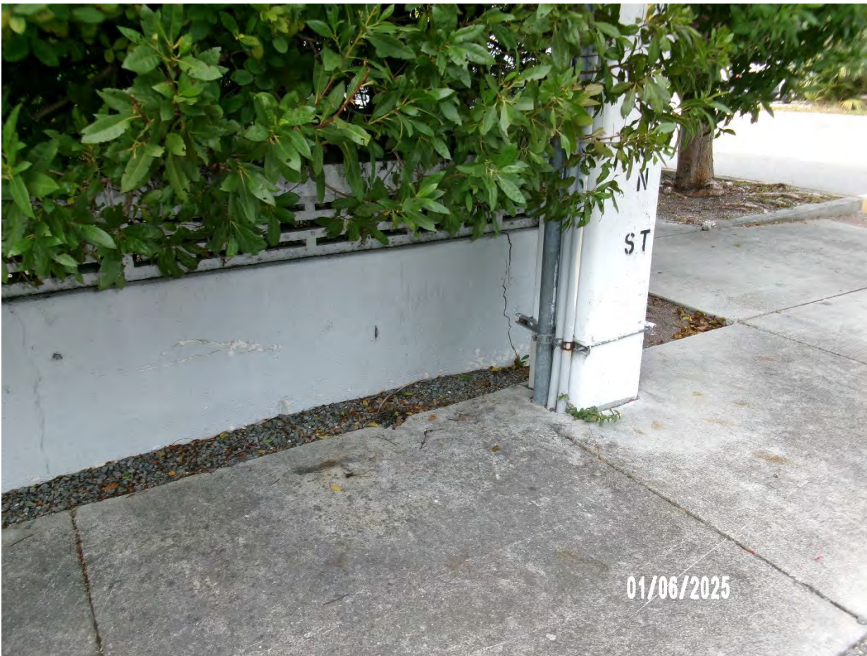
Photo of cracked wall at corner of property, away from tree.
