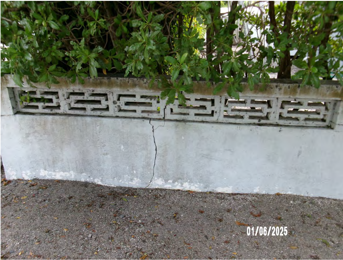
Photo of cracked wall on Flagler side of property. Tall buttonwood shrubs exist along the perimeter of this section of the property.
