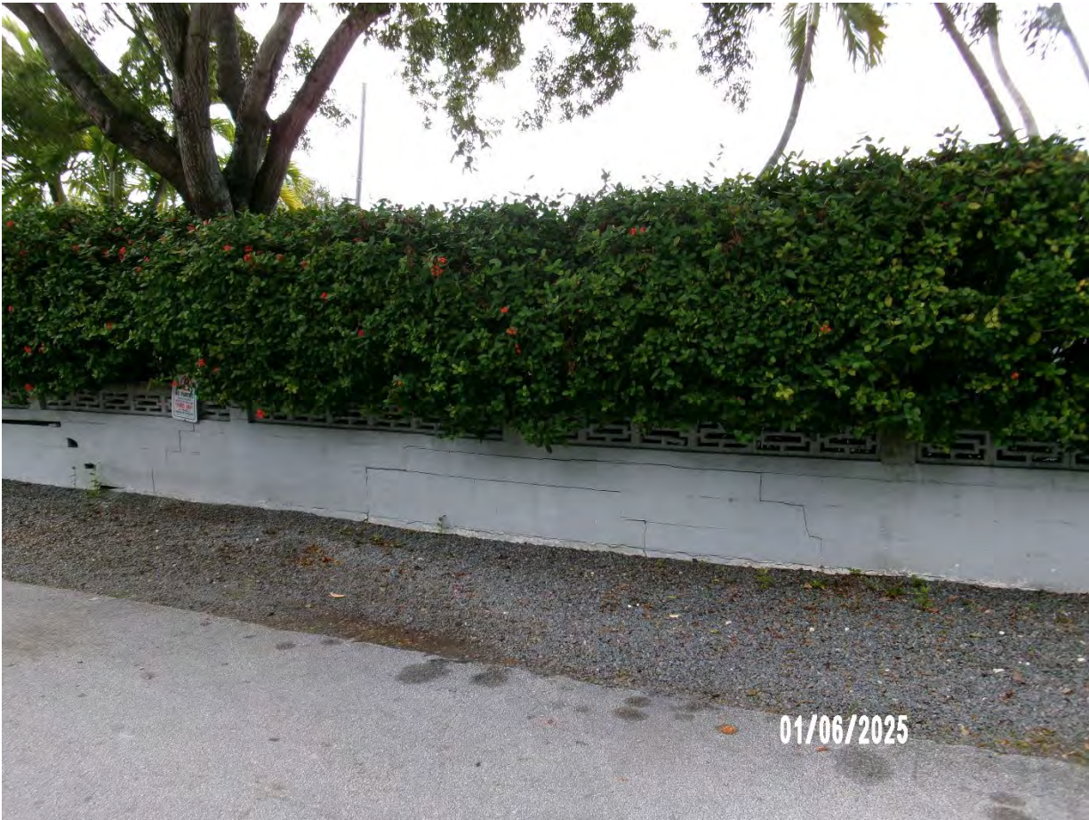
Two photos show tree location and cracked wall.
