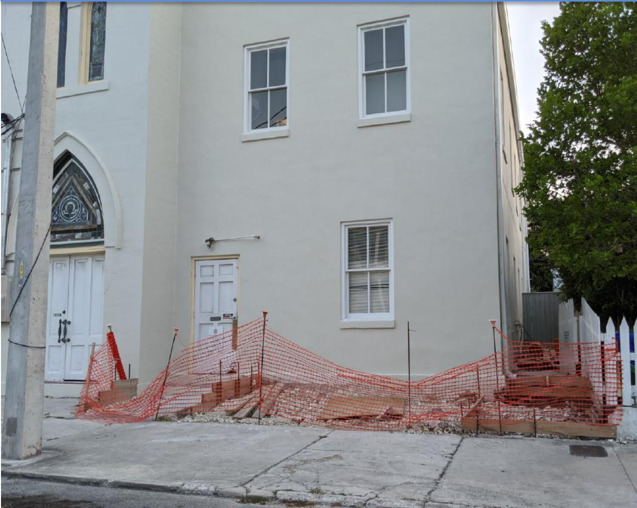
The William Street existing plant bed encroachment will be demolished in order to construct a ADA ramp to the entrance of the church.
