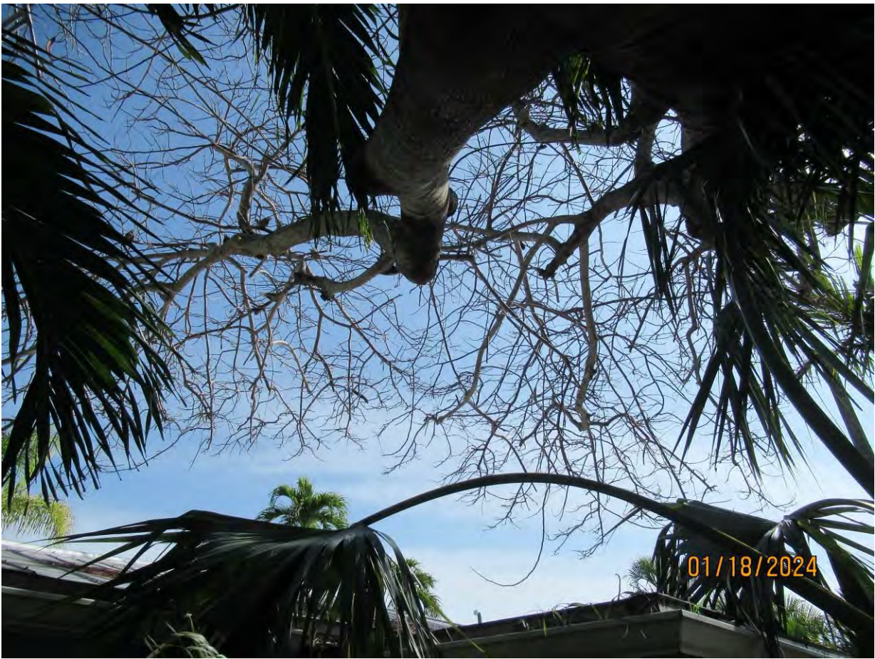
Standing at tree trunk looking at canopy growing over structure.
