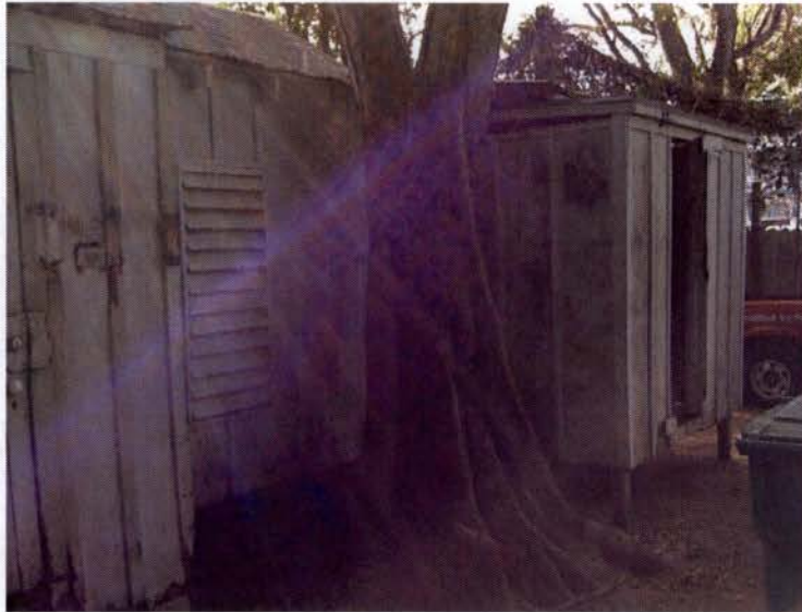
DETERIORATED REAR PORTION OF STRUCTURE TO BE REMOVED
