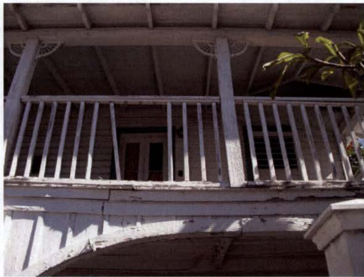
FRONT SECOND FLOOR PORCH, RAILING TO BE REPAIRED
