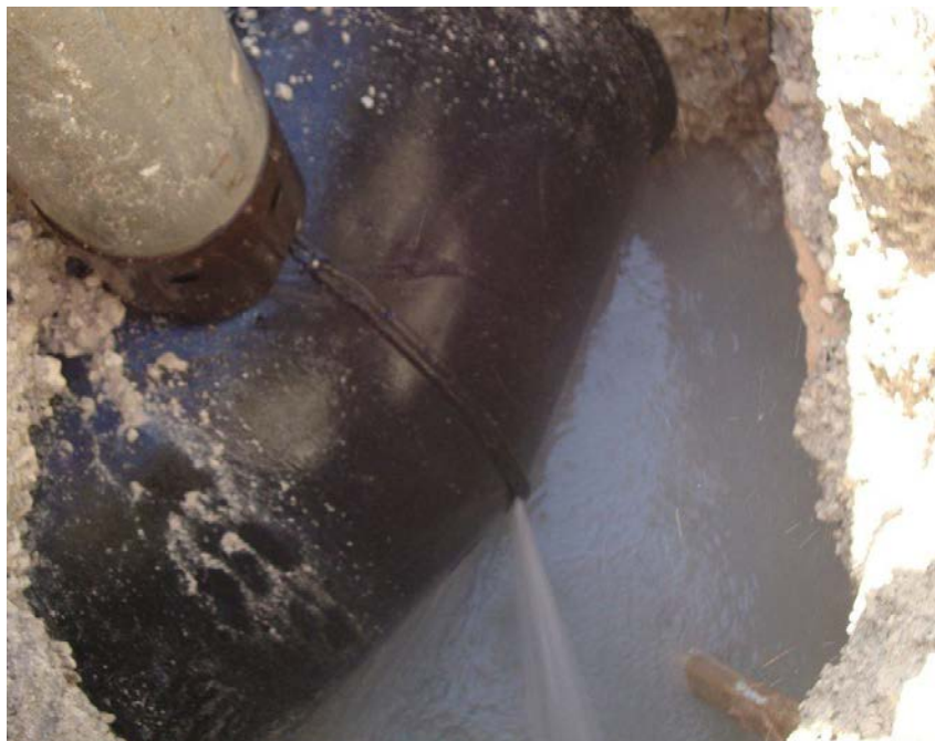
Figure 1: Leak in Fitting Weld
