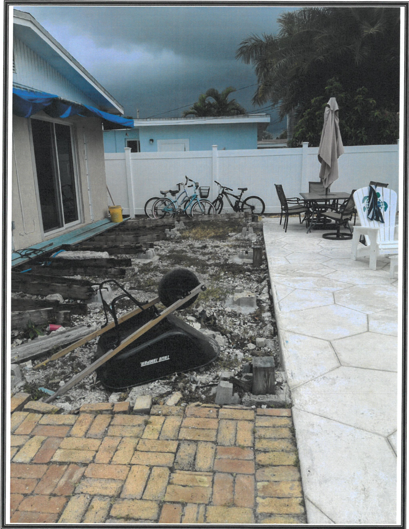
Rear of Principal Structure area where proposed addition and covered porch will be
