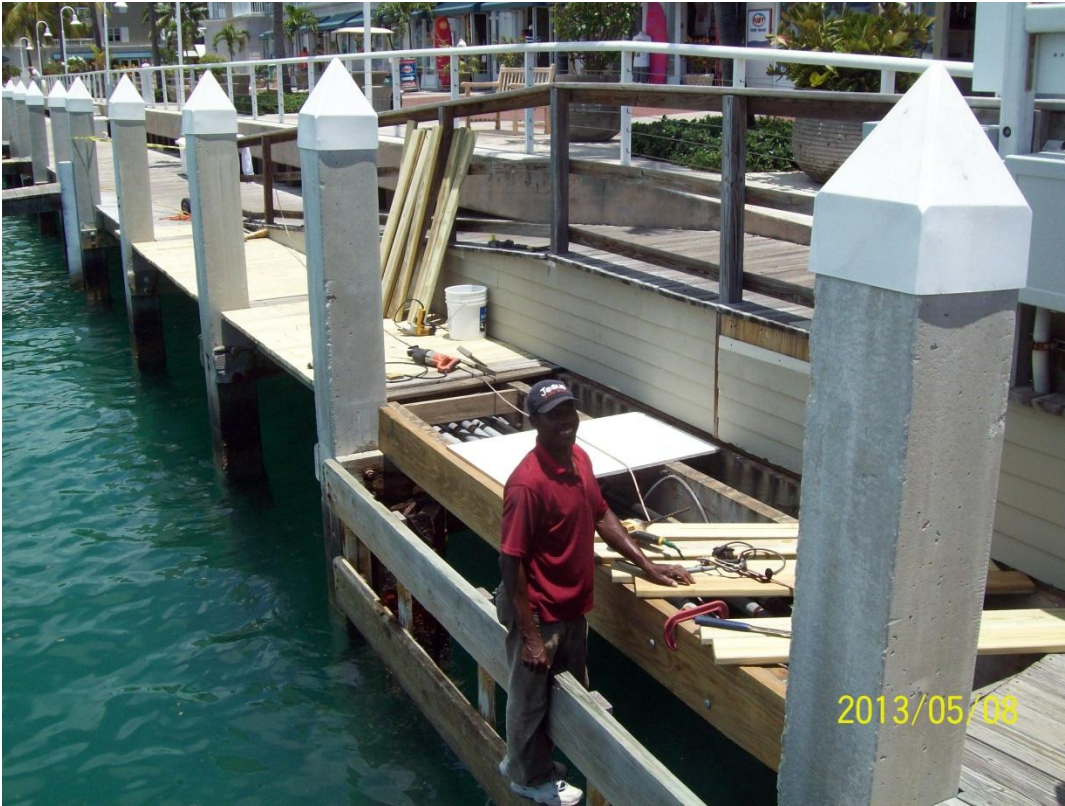
Unpermitted repairs on the pier behind the Westin on 8 May 2013
