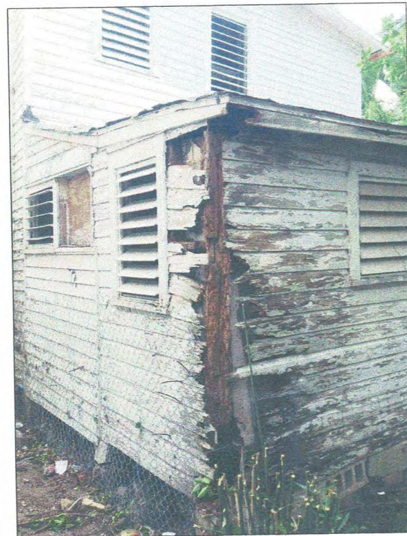
FIGURE 4 REAR VIEW OF DAMAGED ADDITION
