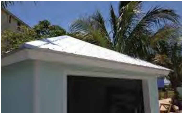
Low Slope Shed Roof over bathroom: Liberty Self Adhering - white in color
