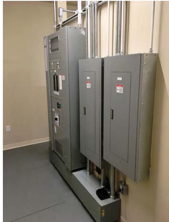
Electrical Panels at Marathon City Hall
