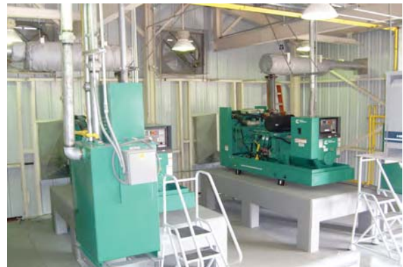
USAF, Generators & Switchgear, Cudjoe Key, FL
