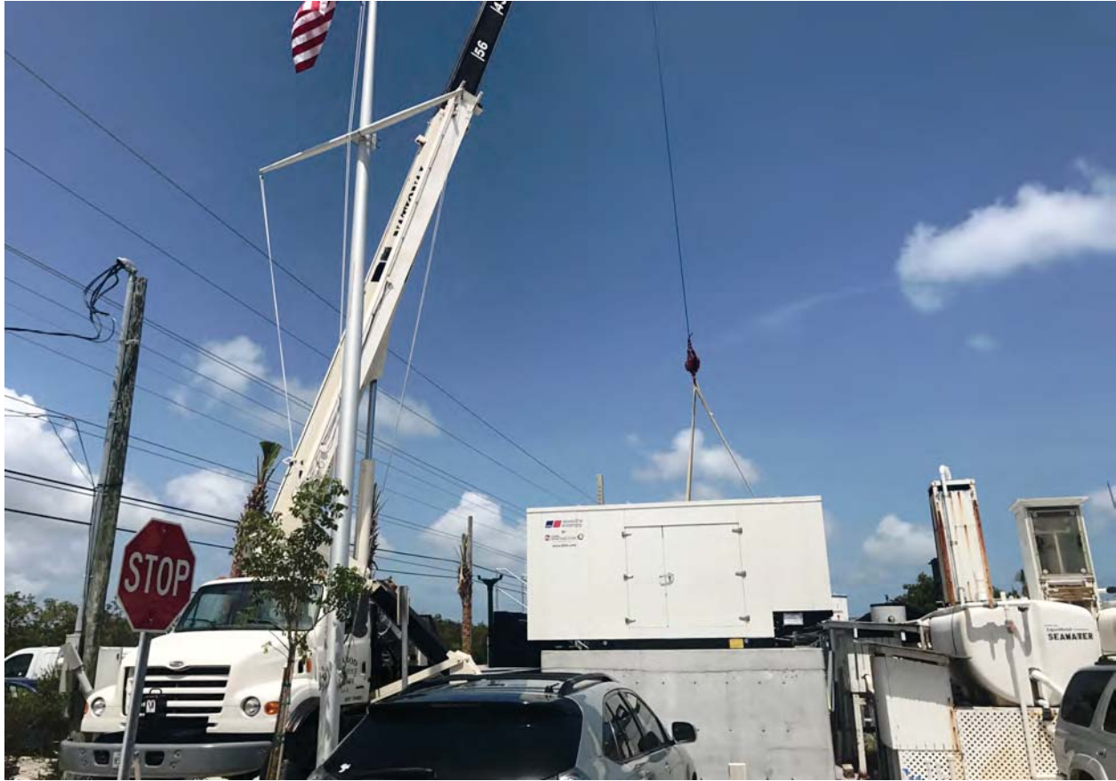
Generator Installation at Mote Marine Tropical Research Lab, Summerland Key, FL
