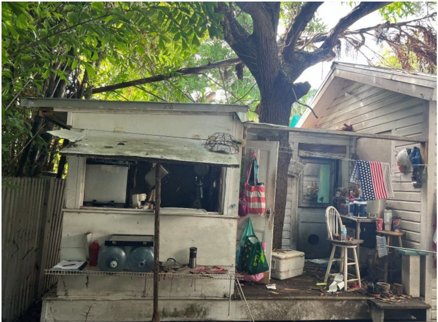
Side and rear view of current accessory structure proposed to be demolished.
