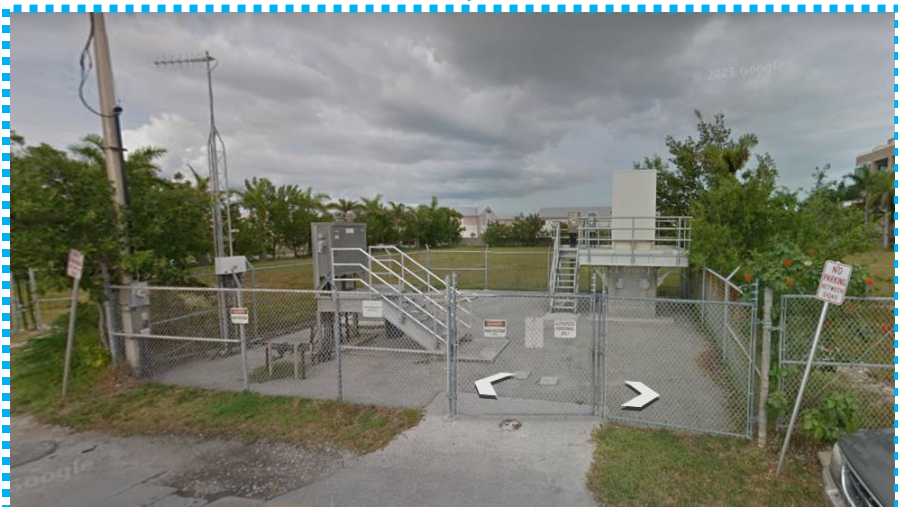
2. The existing water pump/lift station will remain on-site, and significant landscaping is proposed to enhance the frontage of the property along Trumbo Road.
