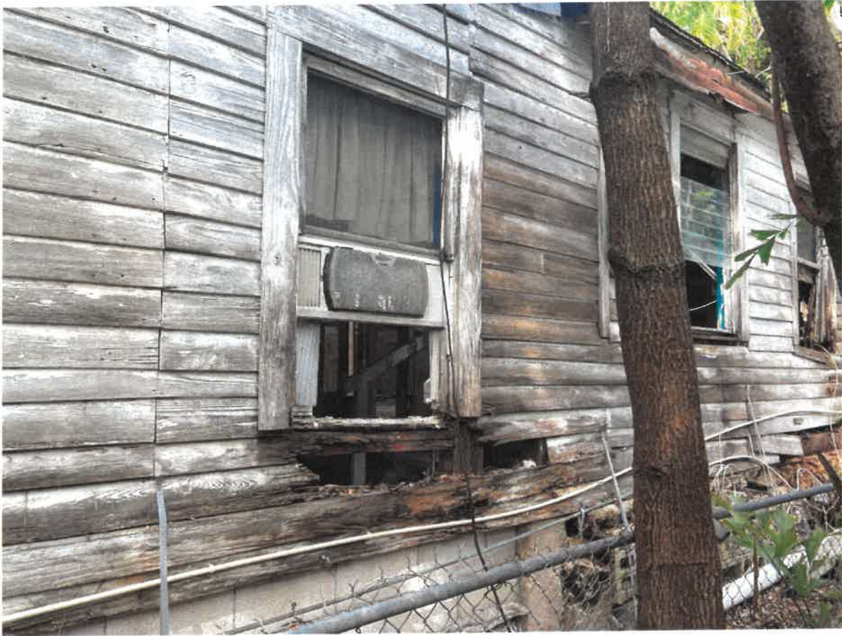
Photograph 7: Photograph of the rotten siding, windows and foundation.
