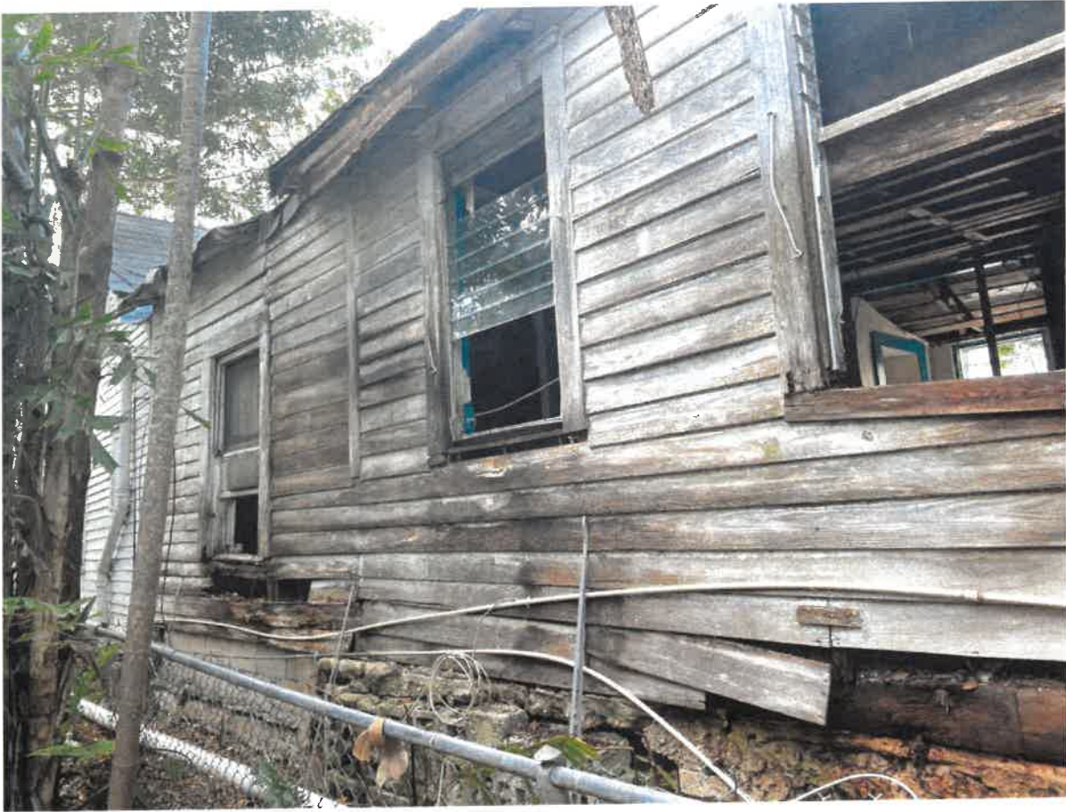
Photograph 5: Photograph of exterior showing damaged windows and rotten siding.
