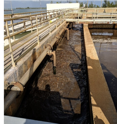
Figure 4-1. MLSS Channel Aeration with Damaged or Missing Diffusers
