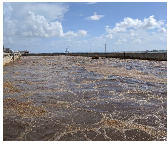
Figure 1-3. Break in Grid in Aerobic Zone 3
