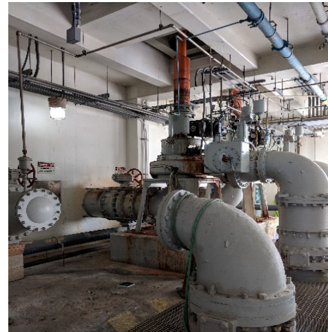
Figure 4-6. Deep Well Pumps with Future Pump Location
