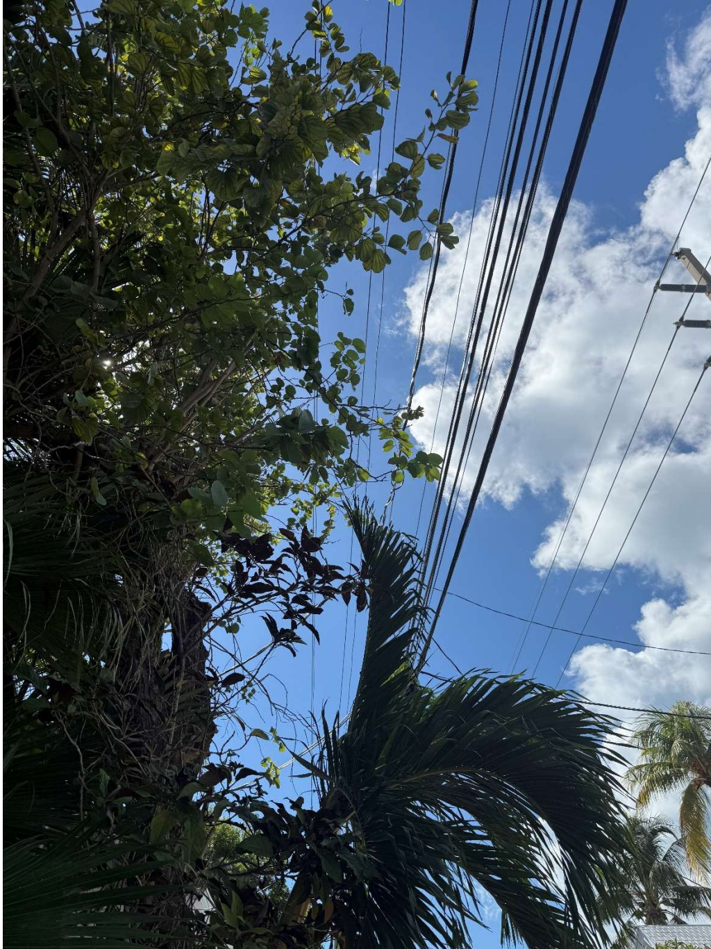
Tree is growing into wires.
