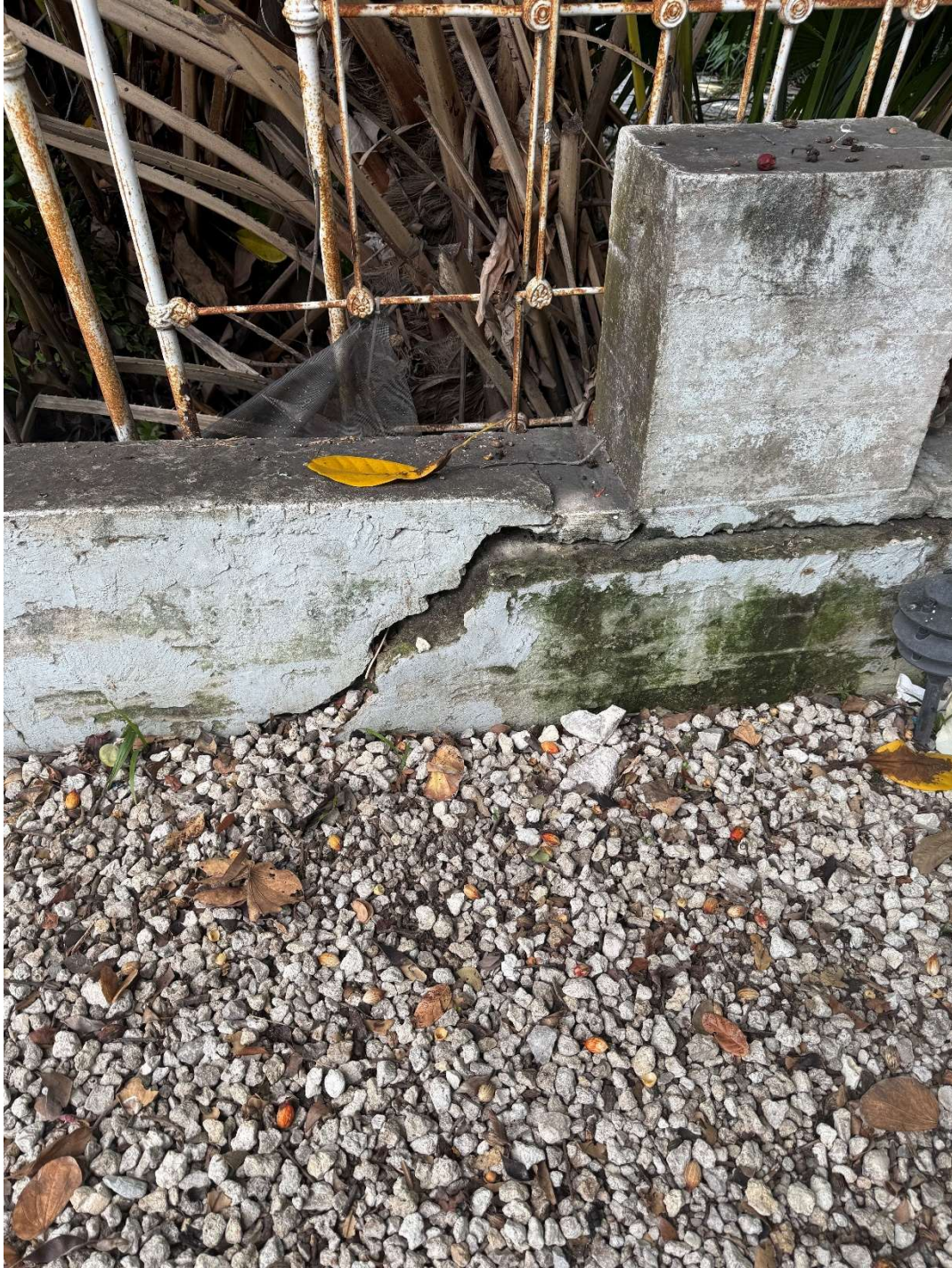
Roots have impacted the wall.
