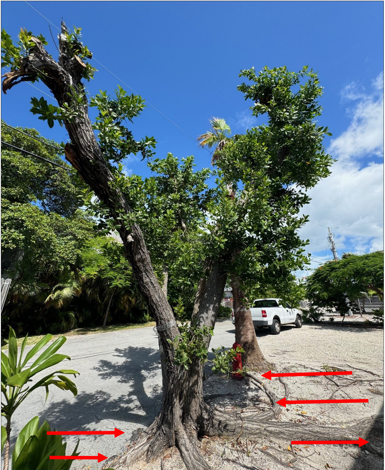
The roots are actively growing into the street, around the fire hydrant and have gone completely under the residence at 3310 Donald.
