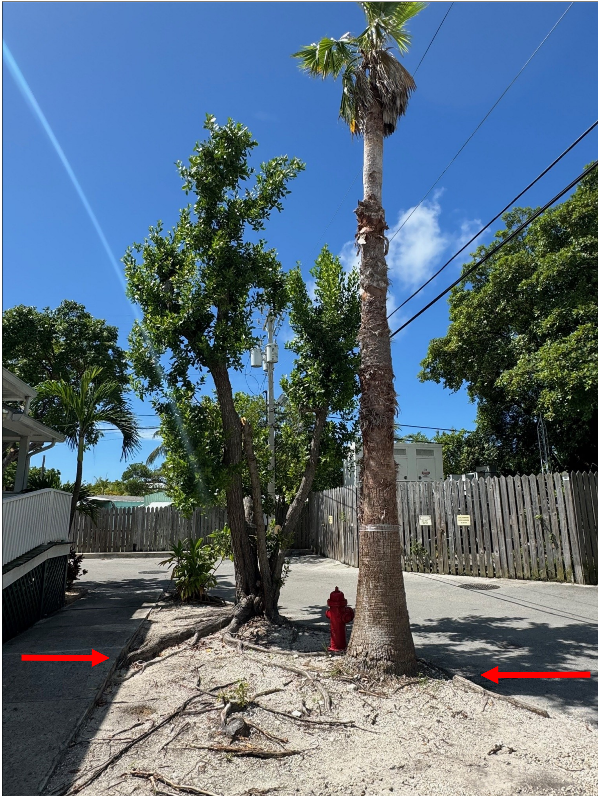
Larger root has lifted the sidewalk.
