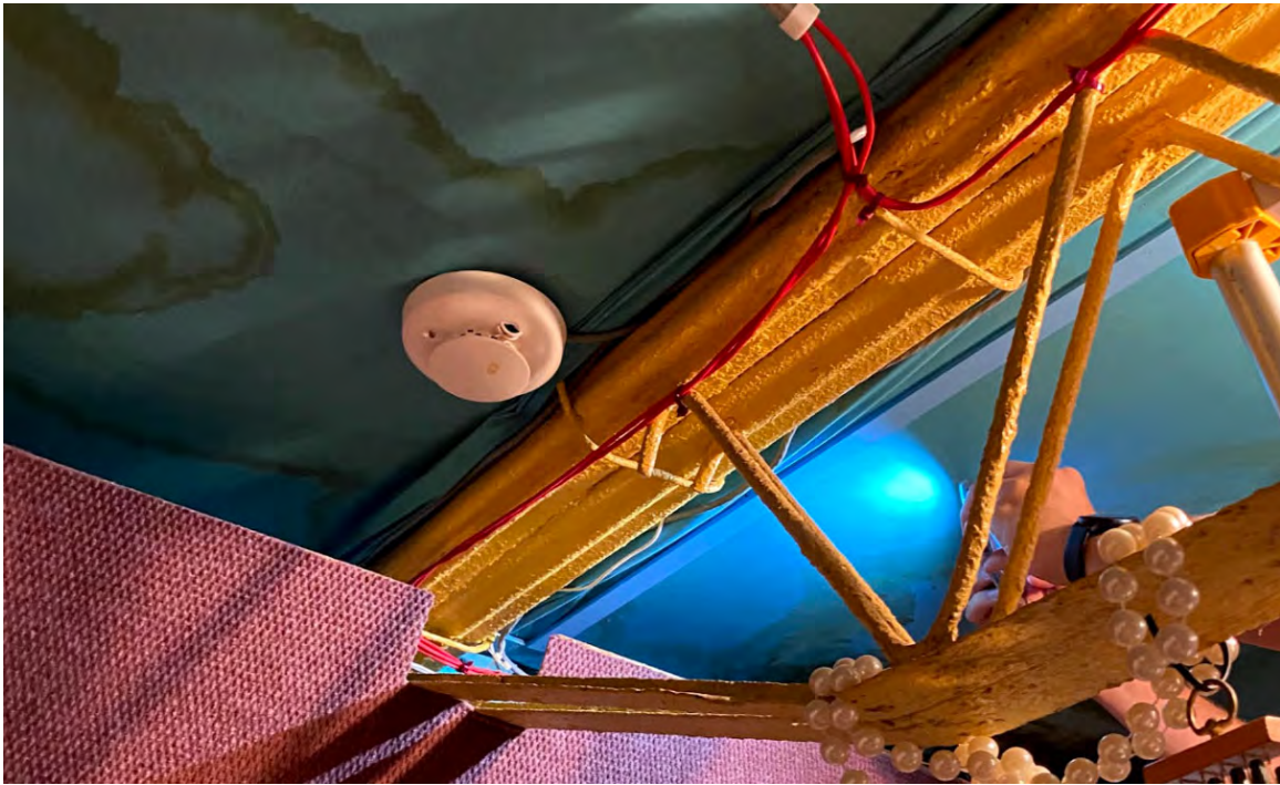
Figure 11. Main Building - Interior view. Existing truss support point over damaged tie-beam.
