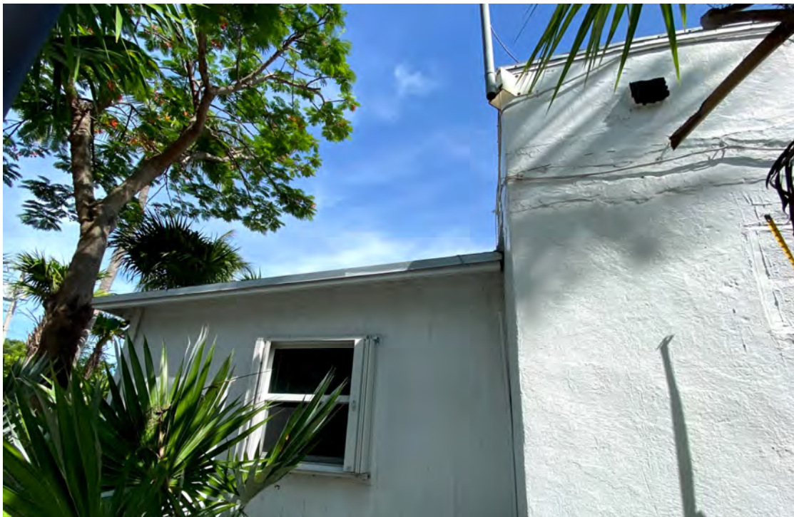
Figure 3. Partial Rear Elevation. Visible concrete damage – cracks along tie-beam.
