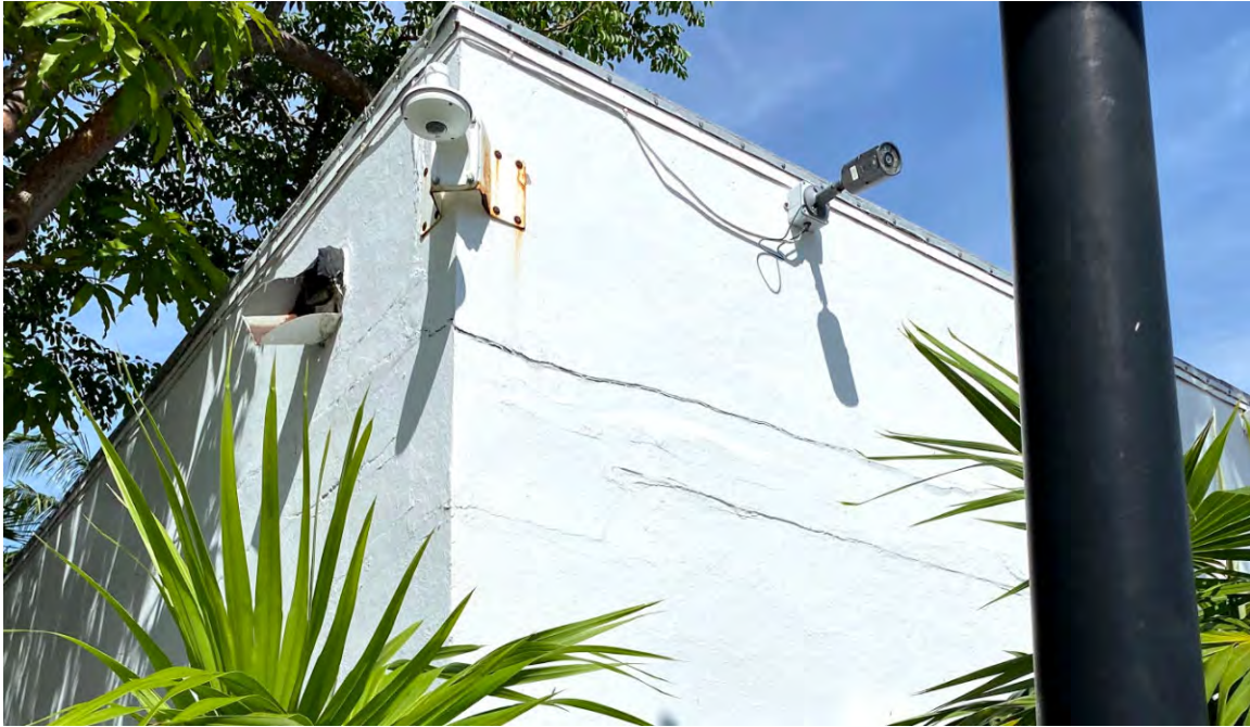
Figure 4. Partial left side elevation. More cracks in the tie-beam.
