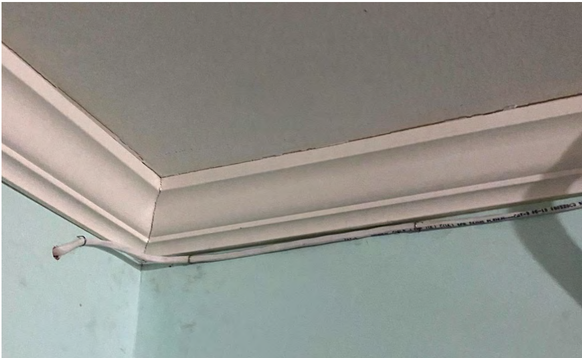
Figure 11. Addition to main building – Visible ceiling cracks along CMU wall. The addition is leaning away.
