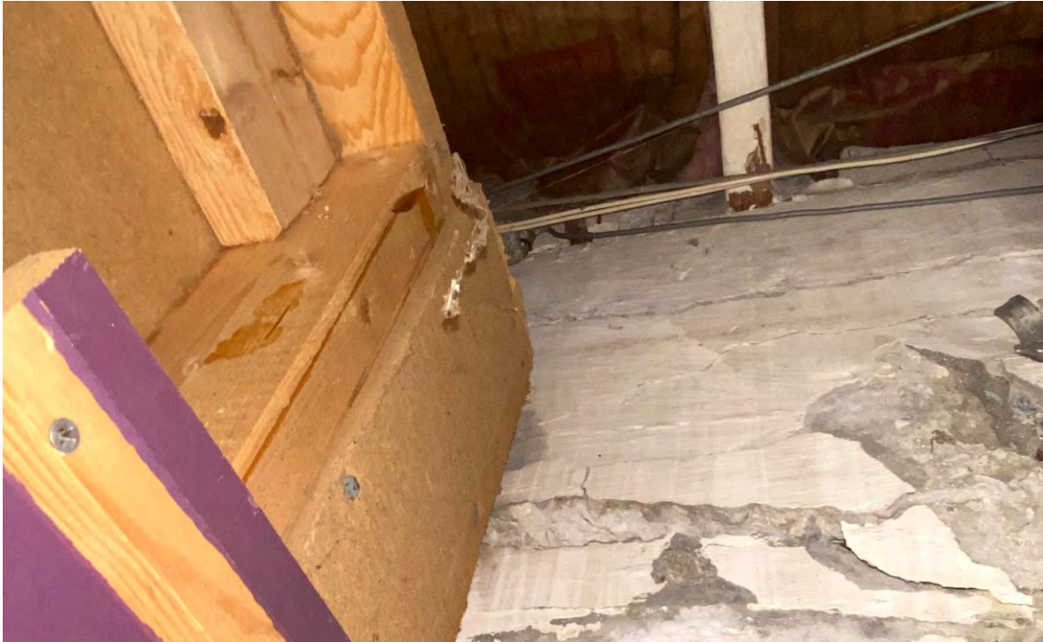
Figure 13. Main Building - Interior view with failing tie-beam.
