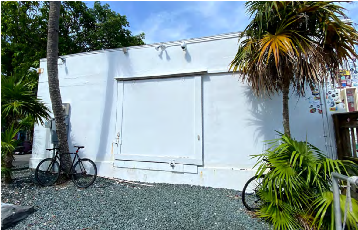
Figure 5. Left side elevation. Tie-beam with damage above decorative sliding doors.
