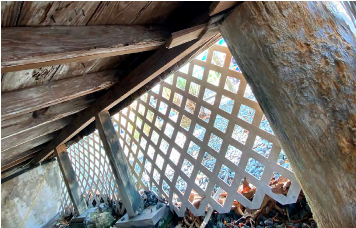
Figure 14. Addition to main building – Heavy damage of wood frame floor system. Perimeter sill beam is completely gone, and floor is supported by temporary shoring. Inadequate repairs of floor joists.
