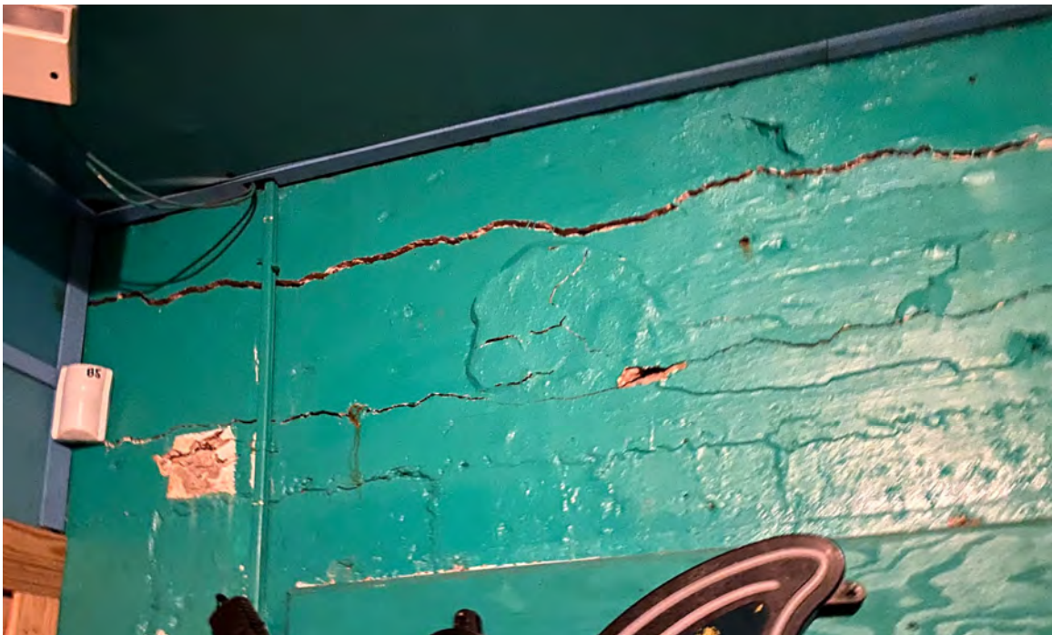
Figure 9. Heavy concrete damage, damaged tie beam (interior of the main building). Please note that on interior the cracks were not patched and are fully open.
