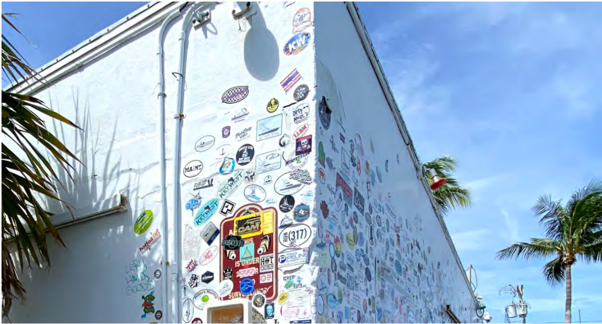
Figure 6. Partial Front Elevation. Tie-beam with damage around the main building perimeter.
