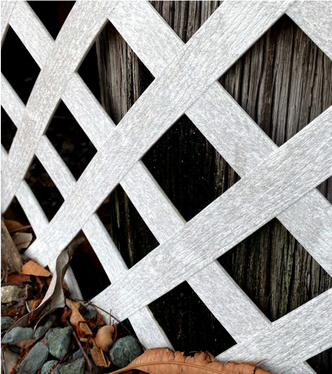
Figure 17. Damaged failing timber pile piers. In need of replacement.
