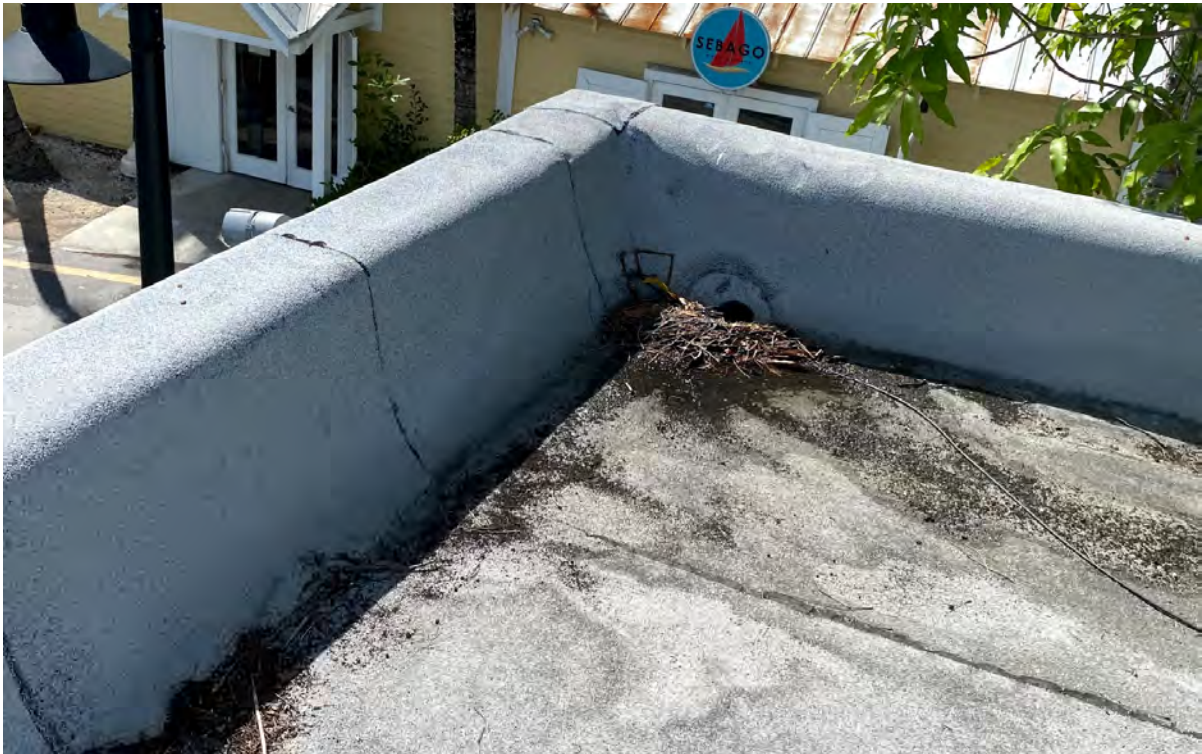
Figure 7. Existing roof scuppers are +/- 4" round pipe and undersized. Debris is clogging the drains and promote standing water along the South-East parapet wall. Recommending upsizing to 8x16 scuppers. Recently reinstalled 3-ply roofing is acceptable condition, however there is no sufficient pitch from the middle of the roof to the side scuppers and some standing water will remain and decrease roofing longevity. At the next re-roofing an installation of tapered insulation in form of "cricket" between two scuppers is recommended.
