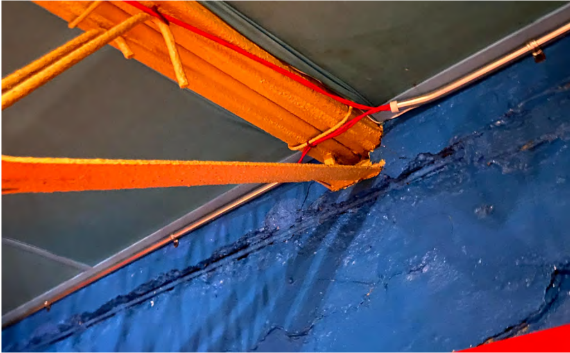
Figure 10. Main Building - Interior view with damaged top of tie-beam at bar joist support. The delaminating (spalling) concrete cover was removed and rebar painted.
