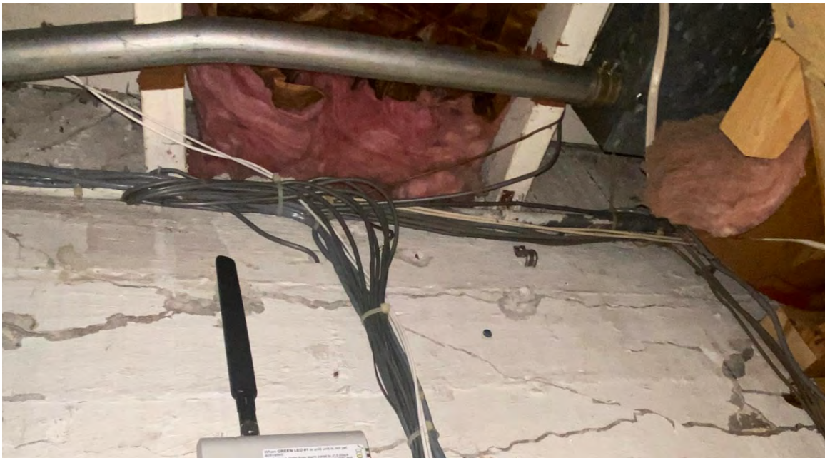
Figure 12. Main Building - Interior view with damaged tie-beam. Misc. damage to roof rafters by electrical conduit pipe.
