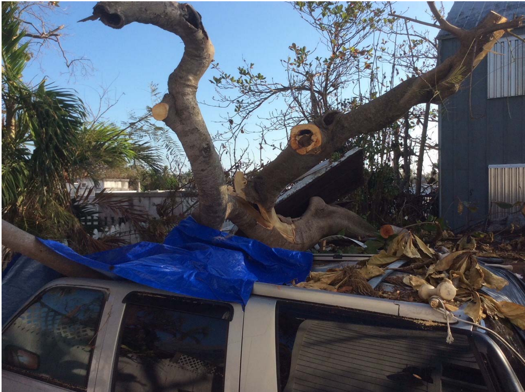
805 Olivia Street, Key West, Florida 33040 HURRICANE IRMA DAMAGE TO EXISTING NON-CONFORMING STRUCTURE
