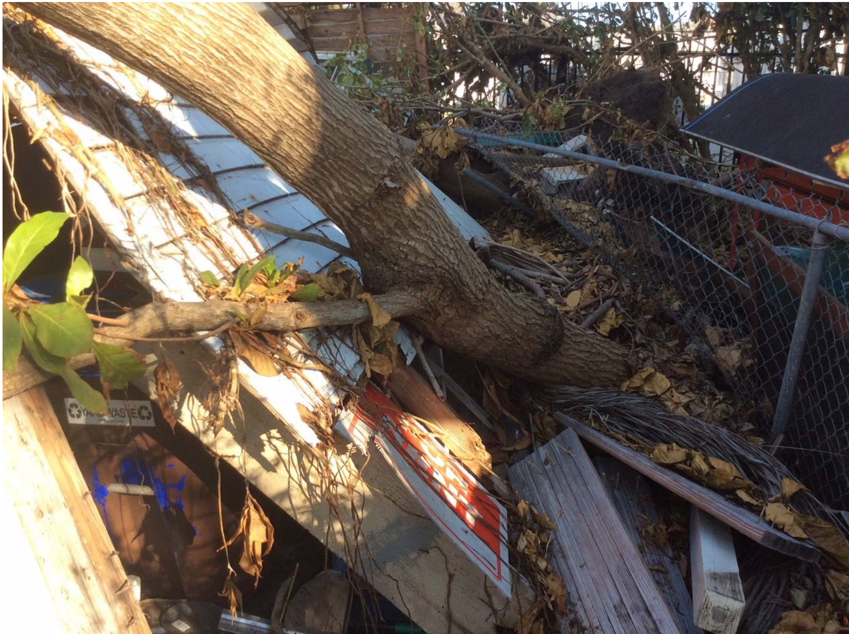
805 Olivia Street, Key West, Florida 33040 HURRICANE IRMA DAMAGE TO EXISTING NON-CONFORMING STRUCTURE
