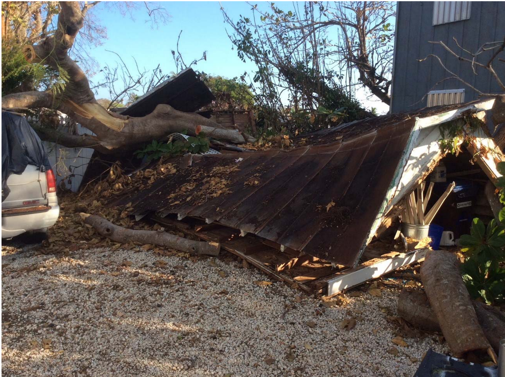
805 Olivia Street, Key West, Florida 33040 HURRICANE IRMA DAMAGE TO EXISTING NON-CONFORMING STRUCTURE
