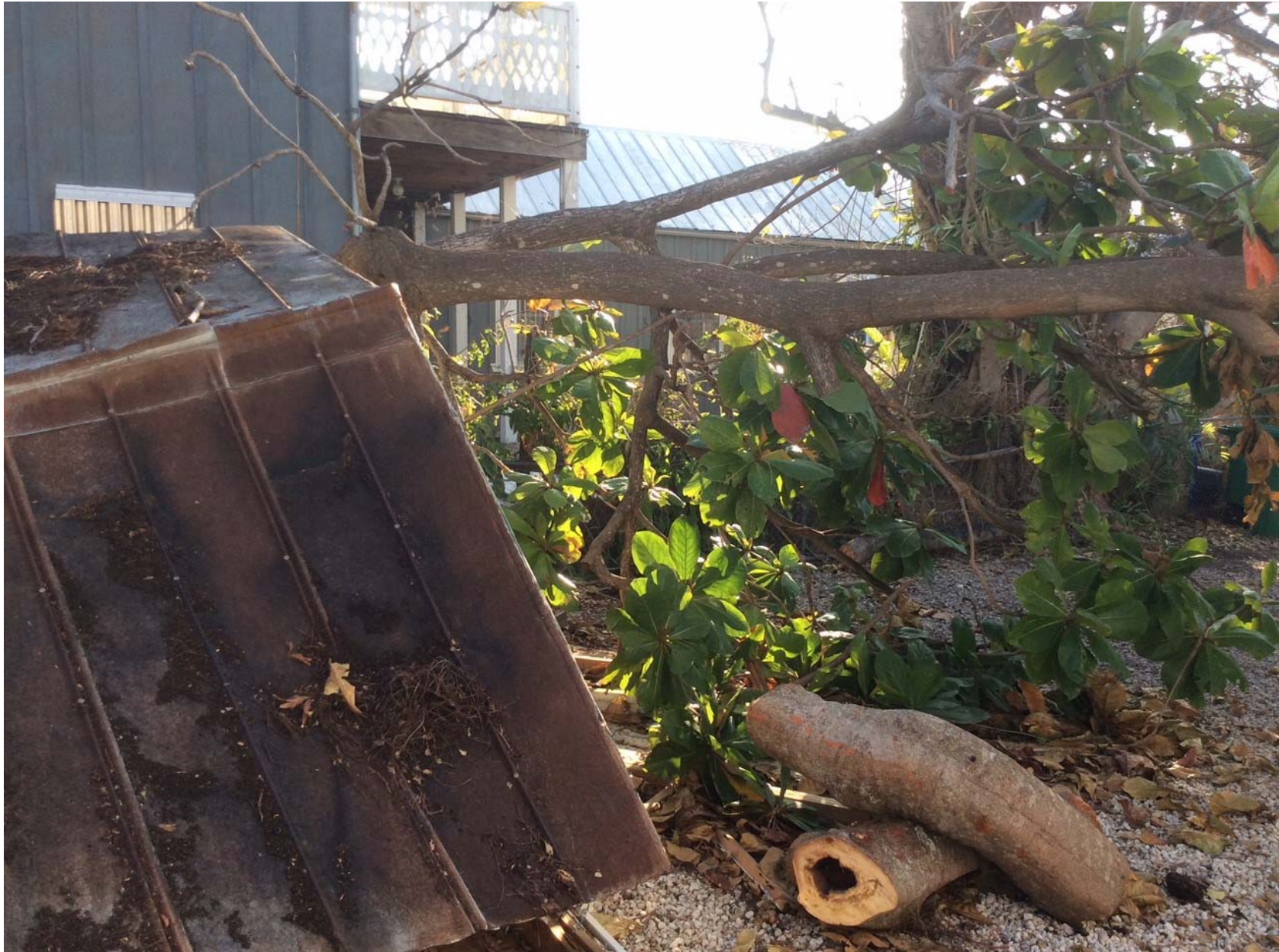
805 Olivia Street, Key West, Florida 33040 HURRICANE IRMA DAMAGE TO EXISTING NON-CONFORMING STRUCTURE
