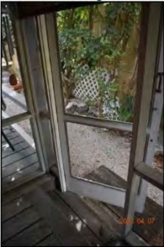
Screened door functioned properly.
