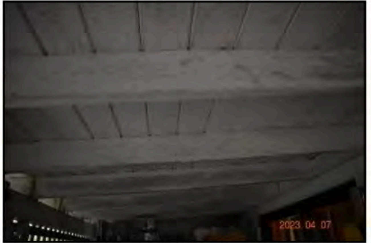
Porch ceiling was secure but weathered.
