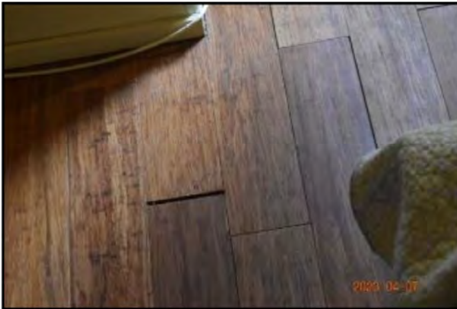
Section of flooring was separated.
