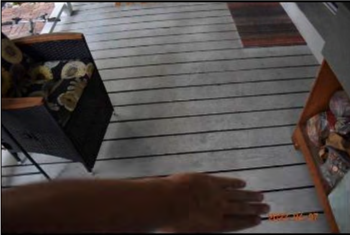
Rear porch sloped towards structure (most likely due to tree roots).
