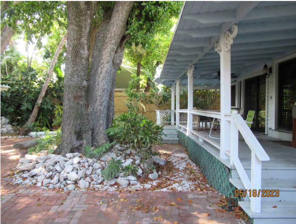
Photo showing location of base and trunk of tree related to the structure, view 2.
