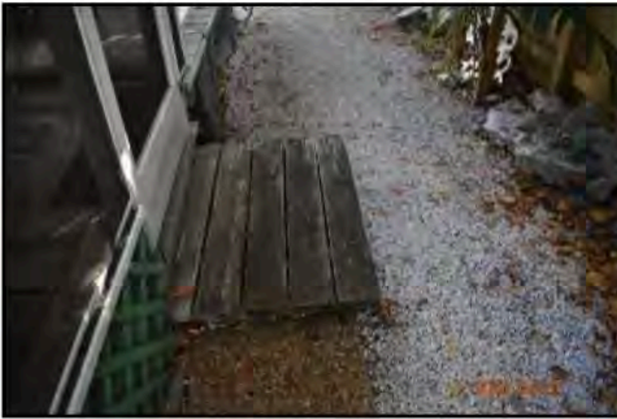
Step was deteriorated.
