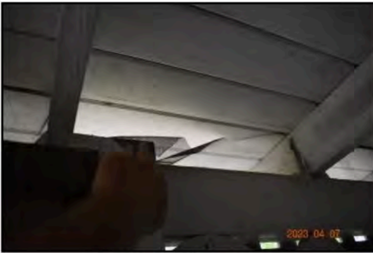
Porch screening was torn.
