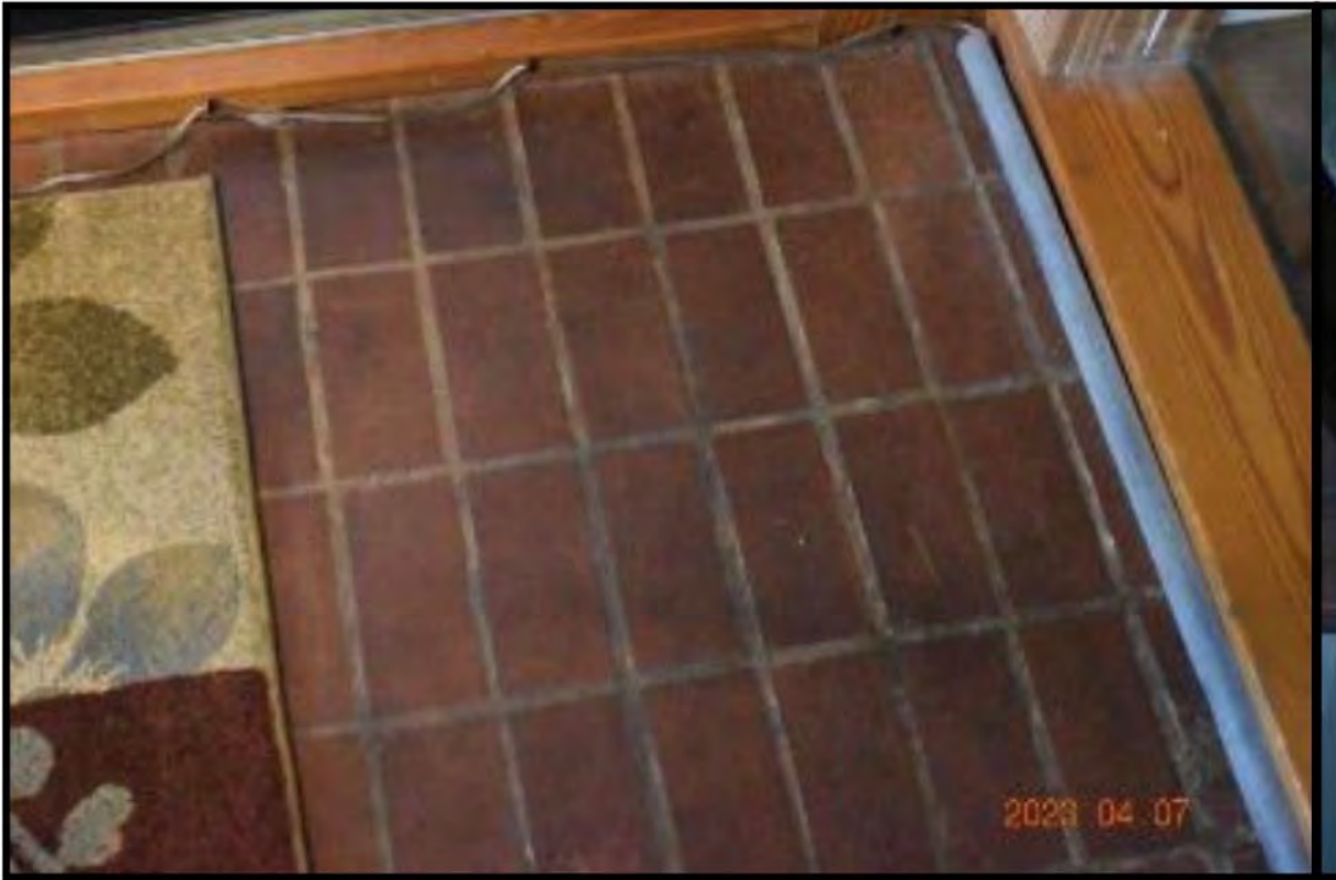
Brick flooring in living room area was worn and sloped.
