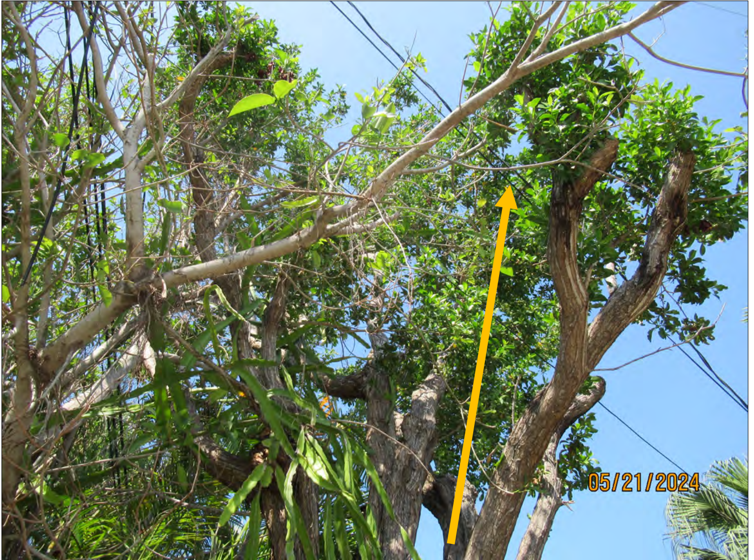
Green buttonwood tree canopy is growing into the utility lines.
