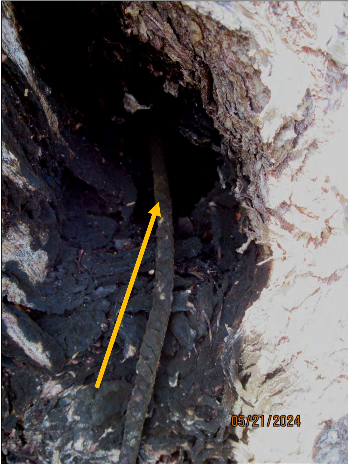
Back side of cavity that is a result of tree bracing materials never removed.
