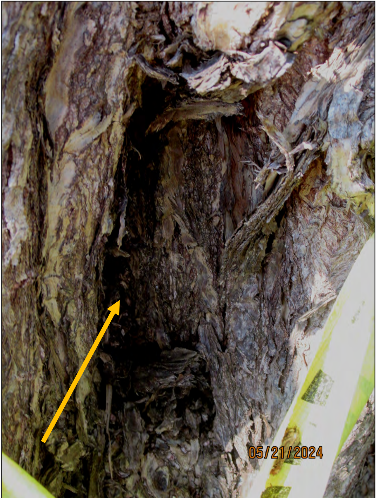
Additional cavity on trunk from improper cuts through the branch collar, making it impossible for the tree to produce wound wood.
