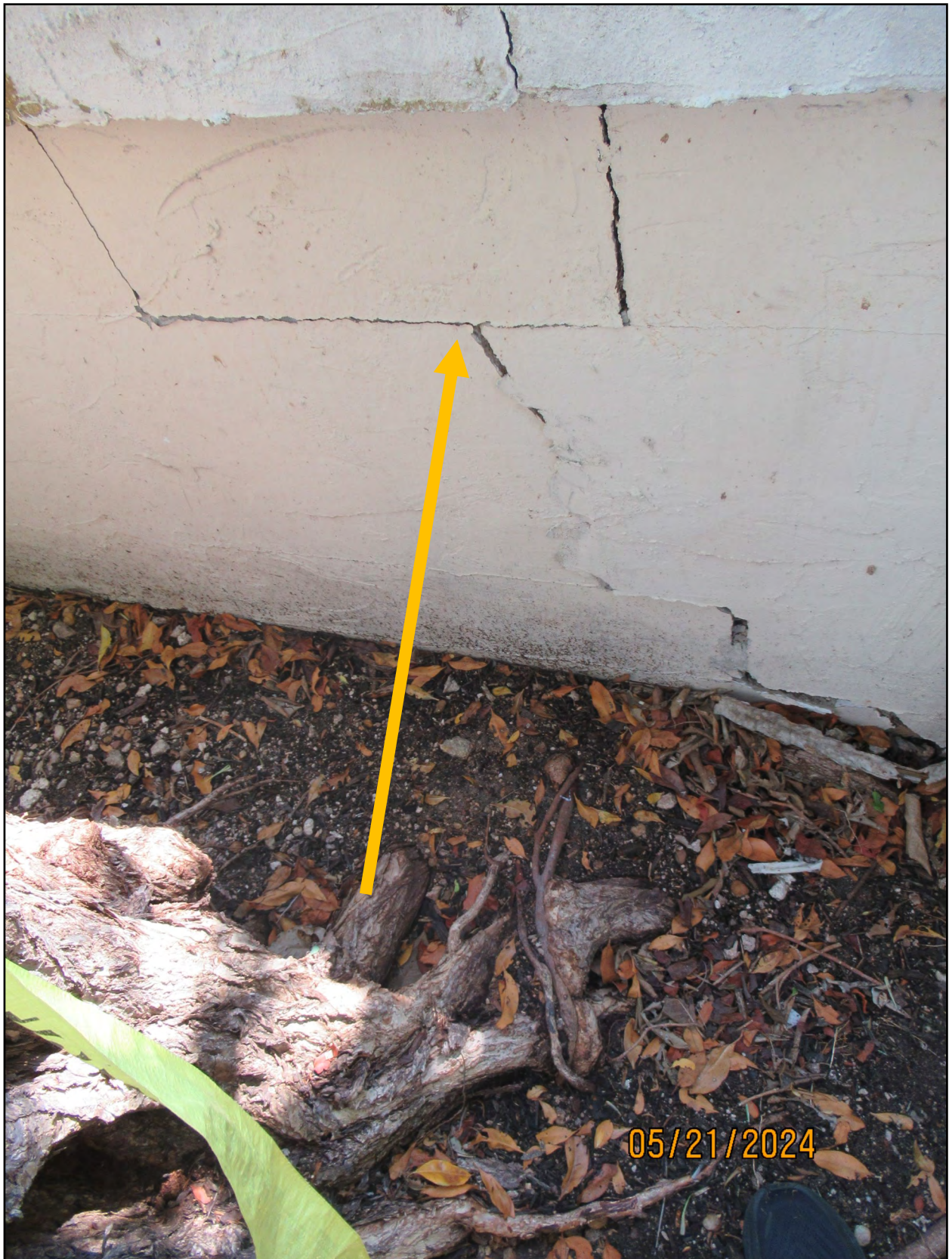
Stair-step cracking of the retaining wall on the property line.
